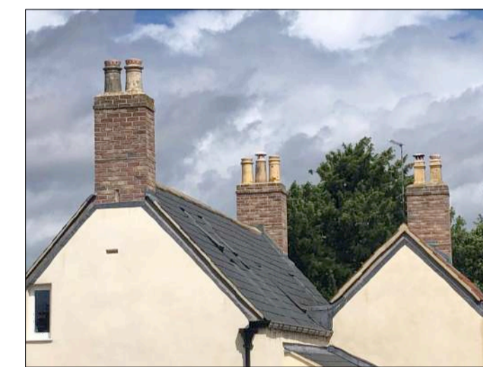
PHOTO 1: 3no. RE-BUILT CHIMNEYS IN BRICK TO MATCH ORIGINAL DESIGN AND WITH RECLAIMED POTS
