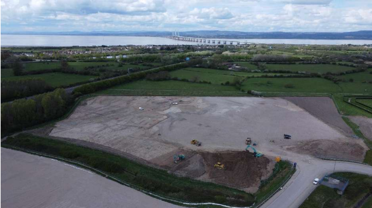
Plate 1: Plot 3 Piling site, located approximately 1.40km east of the Severn Estuary and the M4 Prince of Wales Bridge.
