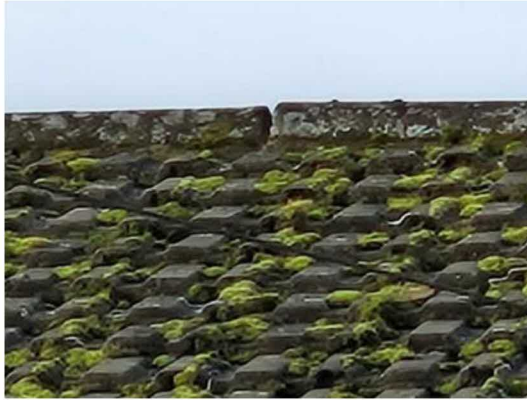
Photograph 10- Potential roost feature 3, missing mortar between ridge tiles
