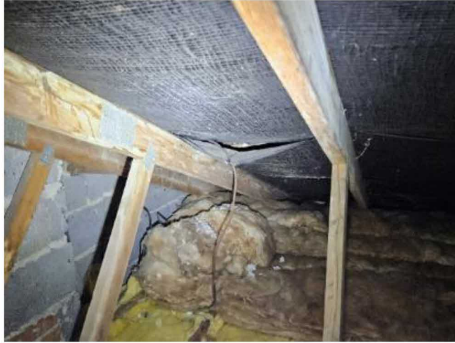
Photograph 7- Potential roost feature 1, gaps between sheets of roofing membrane
