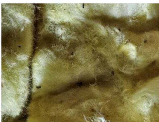
Photograph 15- Mouse droppings in loft
