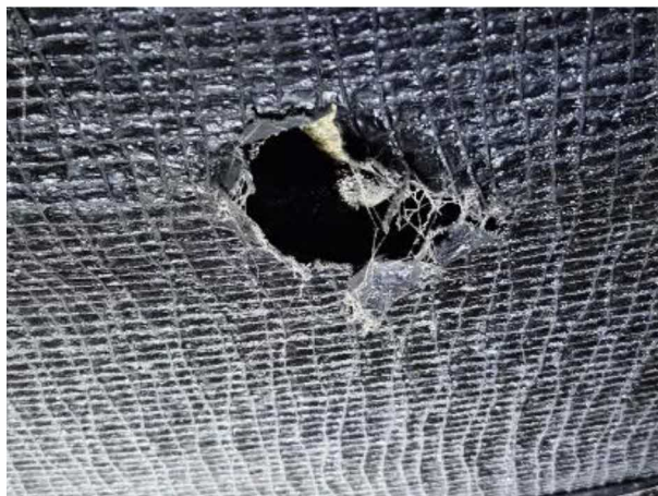
Photograph 6- Potential roost feature 1, hole in roofing membrane
