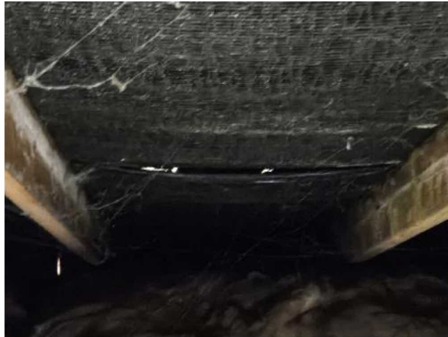
Photograph 5- Potential roost feature 1, gaps between sheets of roofing membrane
