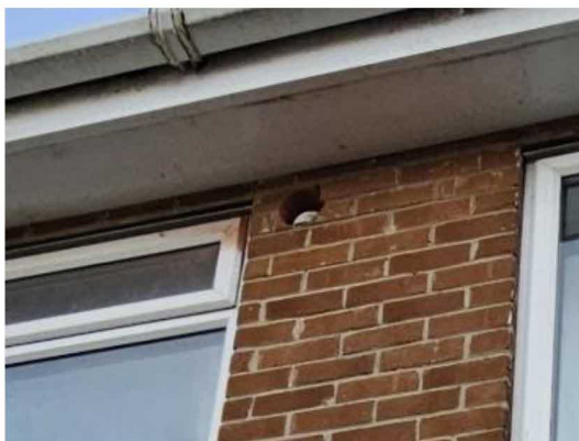
Photograph 13- Potential roost feature 6, hole in brick work on western aspect
