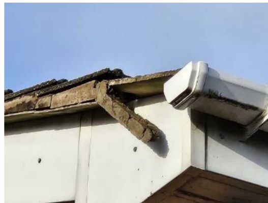
Photograph 12- Potential roost feature 5, missing mortar on southern aspect
