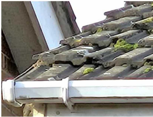
Photograph 11- Potential roost feature 4, lifted roof tiles
