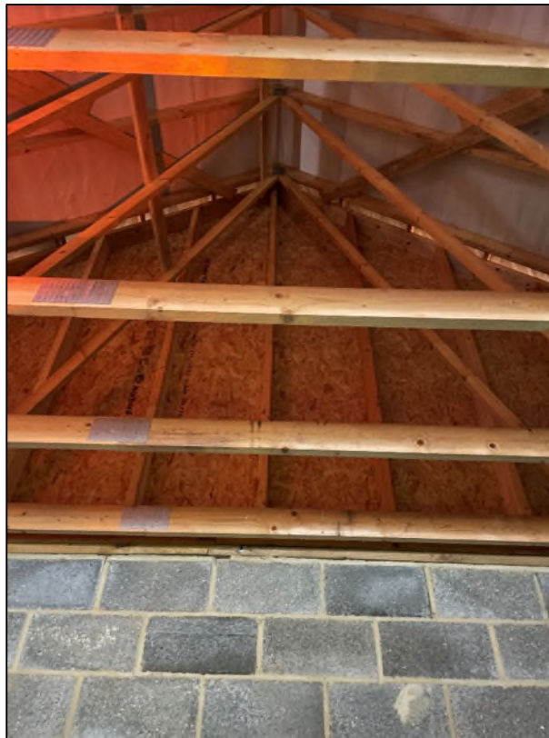
Plate 5: roof structure including chipboard gable end wall, trussed rafters, and breathable membrane lining.
