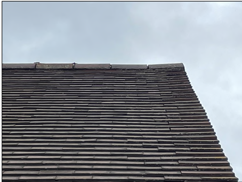
Plate 2: gaps in the mortar of ridge tiles.
