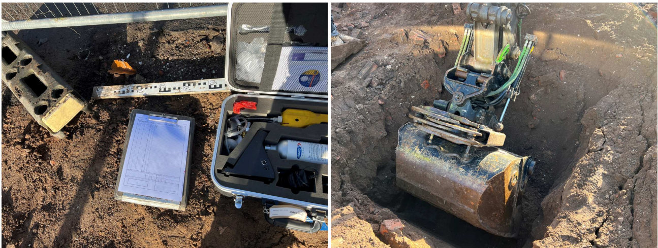
Photographs 3 and 4: Showing the PID equipment used for detecting vapours and the progressive excavation of trial pit TP01 within the location of Tank 1.
