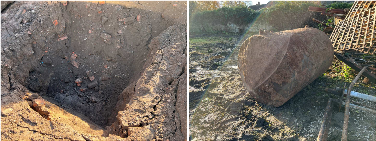
Photographs 5 and 6: Showing trial pit TP01 and the recovered Tank1 ready for disposal.
