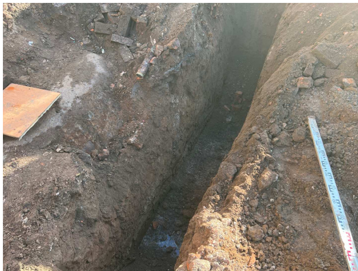
Photograph 7: Showing trial pit TP02 being excavated adjacent to Tank 2 which is left of the photograph.
