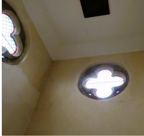
Windows on top floor of north tower stairwell – left hand one faces front
