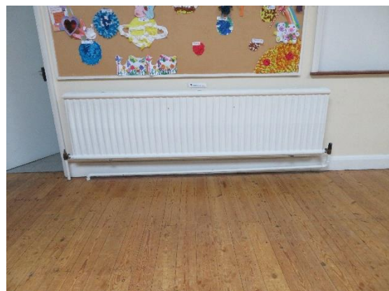
Radiator on kitchen (east) wall
