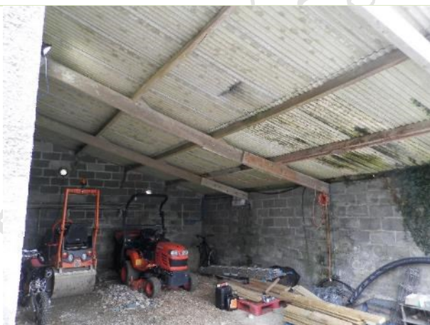
View of the northern half of the barn showing how bright the structure is during the day.
