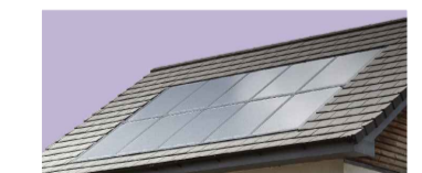
7. PV roof panels
