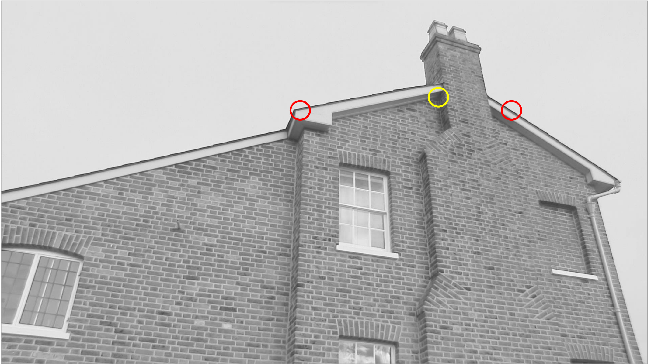
Northern Gable End - from left to right: Brown long eared exit from underneath roof tile (red), brown long eared maternity roost main exit under box soffit on left hand side of chimney (yellow), soprano pipistrelle exit from underneath roof tile to right hand side of chimney (red). Locations are approximate.
