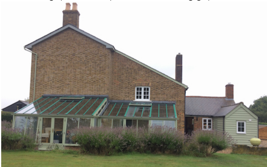
Bats have been noticed exiting from the roof on this elevation
