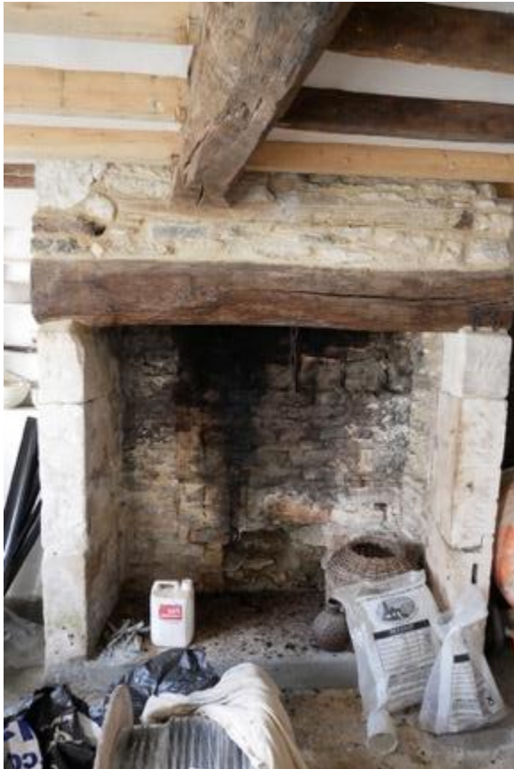
Plate 8: C17 fireplace on east wall with stop-chamfered C17 principal floor beam resting on timber bearer
