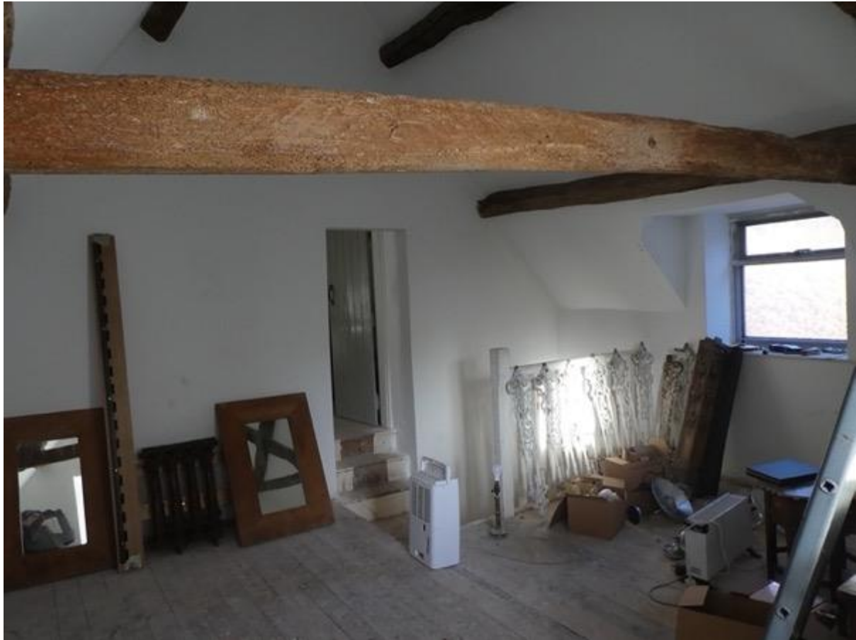
Plate 14: First floor of the C17 section looking west with late C20 staircase, aluminium casement window and C20 plank door to the C19 section
