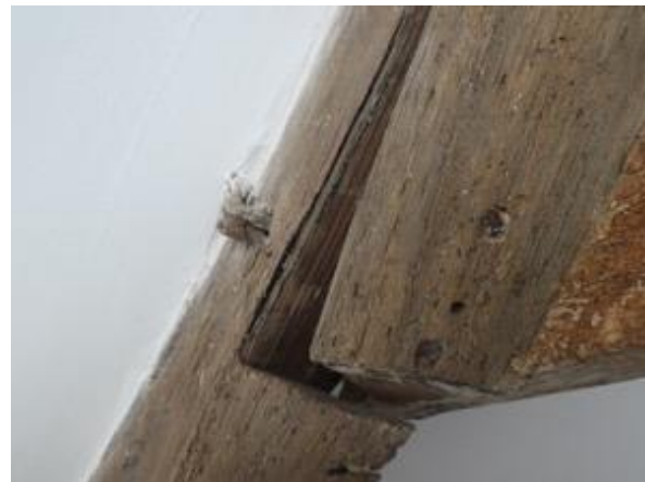
Plate 13: Split principal rafter on south side of truss, the secondary collar is held in place by a wrought iron peg and metal pin and secondary screws
