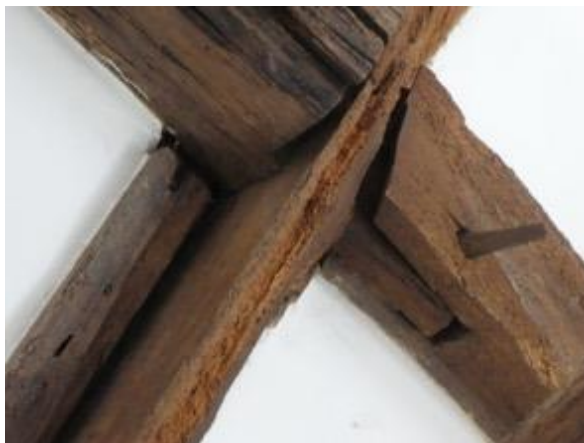
Plate 12: Through purlins have pegged joints in common with the rest of the C17 roof
