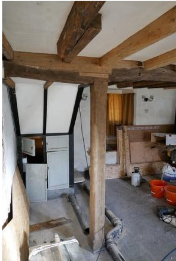
Plate 9: A C20 post supports a joint in the principal floor beam. The beam is flattened suggesting its historical bearing was a partition wall.
