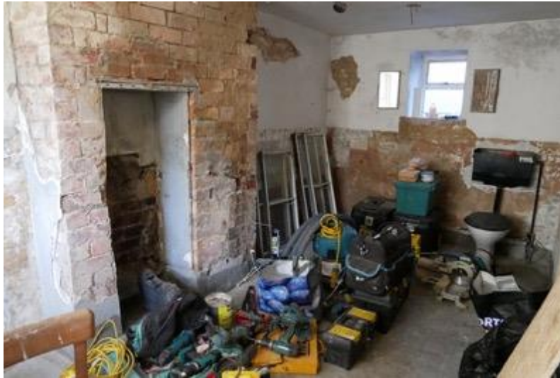
Plate 16: C19 section looking north, brick lined walls and chimney on west gable and C20 casement window
