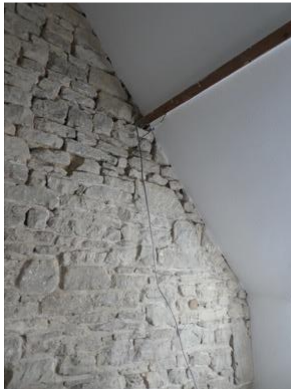
Plate 19: C19 section with C17 eaves line showing in partition wall and C20 purlin
