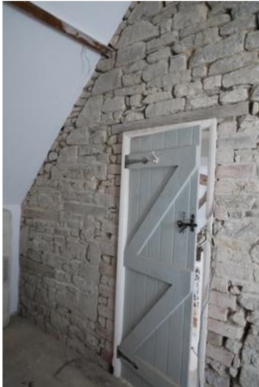
Plate 18: C19 section with rubble stone partition to C17 section right showing former eaves line
