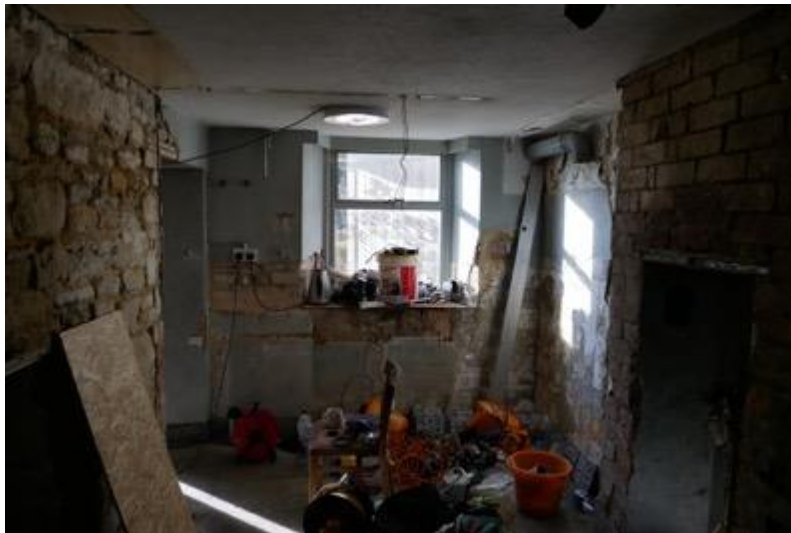
Plate 17: C19 section looking south with rubble stone partition to C17 section left and C20 casement in C19 opening
