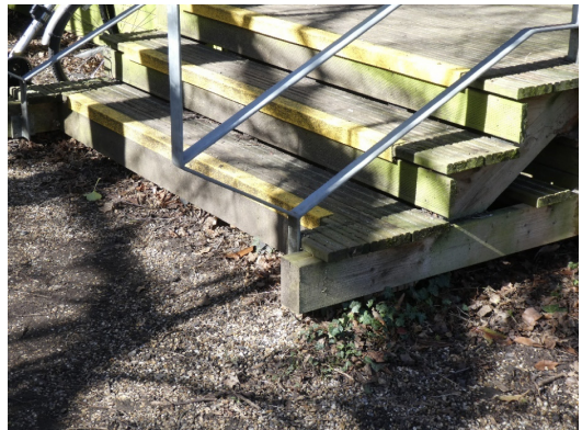
08 Bound gravel will alleviate the problem of ground erosion which has made the entrance to the North Building difficult to access.
