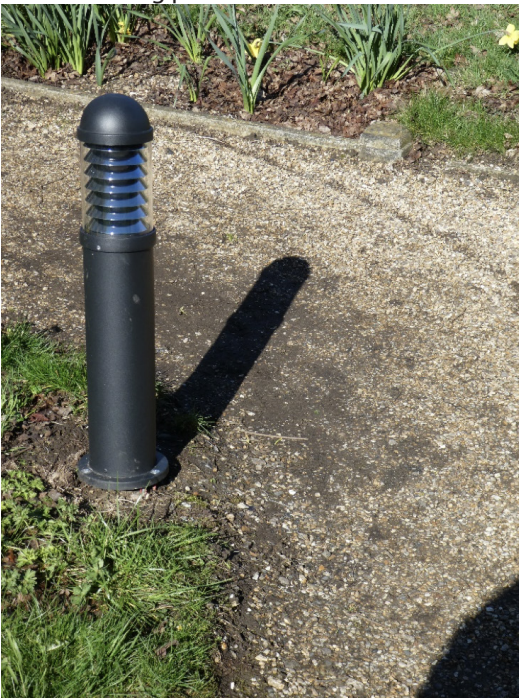
07 additional lighting bollards are proposed along the paths. The external wall light will be removed from the SE corner of the chancel
