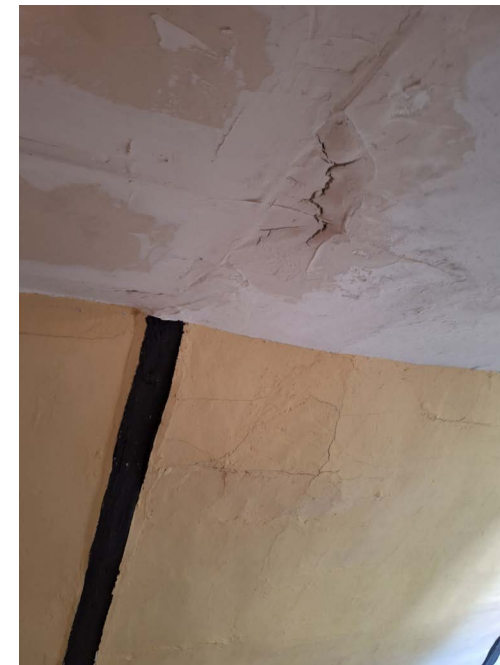
Damage to ceiling on second floor
