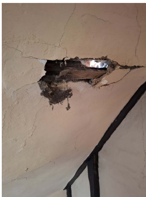
Further damage to ceiling at second floor
