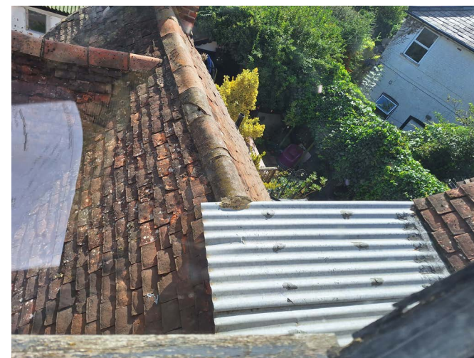
Cemented-in metal sheeting to roof (presumably an ad-hock repair to stop leak & further water damage to Room 7)
