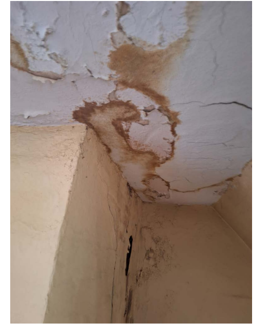
Water damage to ceiling of Room 7
