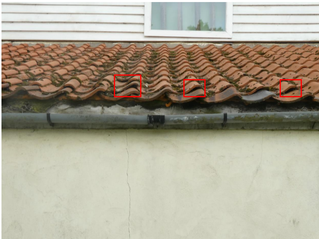
Photo 4 , example of lifted tiles, predominately on the second and third rows of the low-pitched lean-to.
