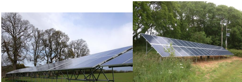
Fig 8. Photos of the previously installed similar solar array.
