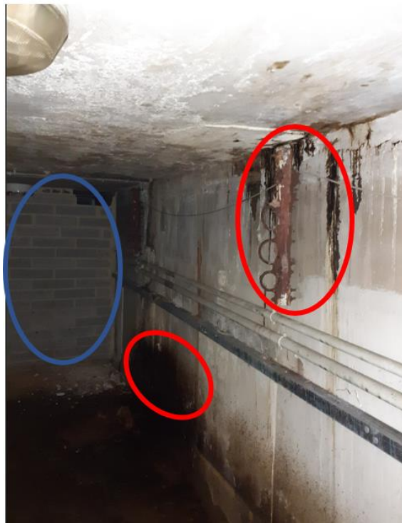
Figure 2.2a Service tunnel with suspected heating oil/kerosene (hydrocarbons)- blue highlights anticipated site boundary and red highlights areas of leakage.
