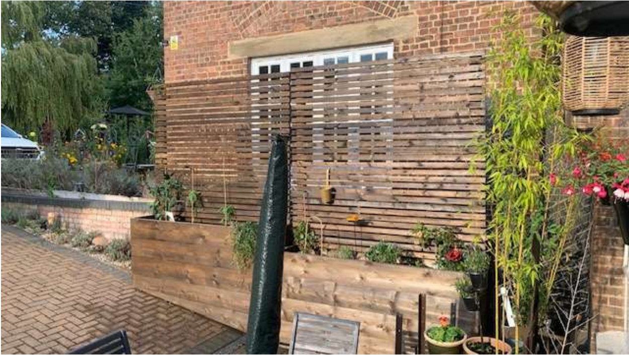
First 2 planters installed. Enforcement visited site and works have stopped since this.
