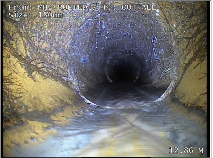
Roots fine, at joint
