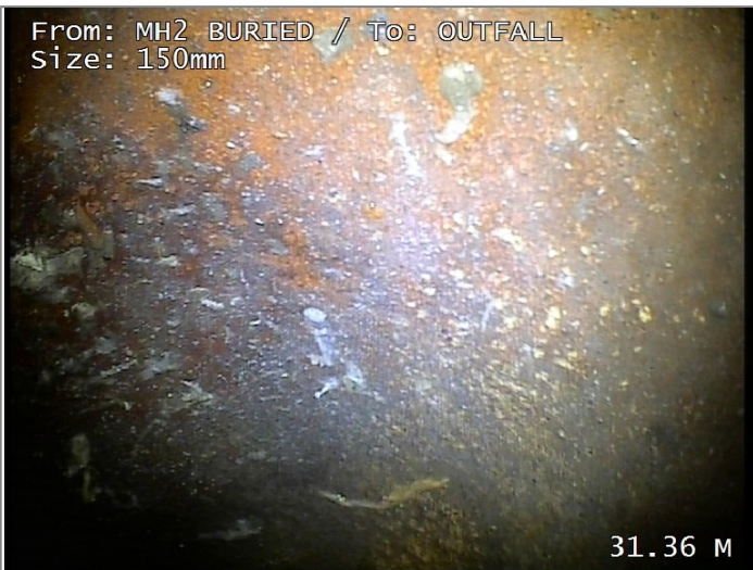
Line of drain/ sewer deviates down
