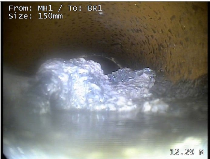
Attached deposits, fouling from 3 to 9 o'clock 50% cross-sectional area loss, at joint
