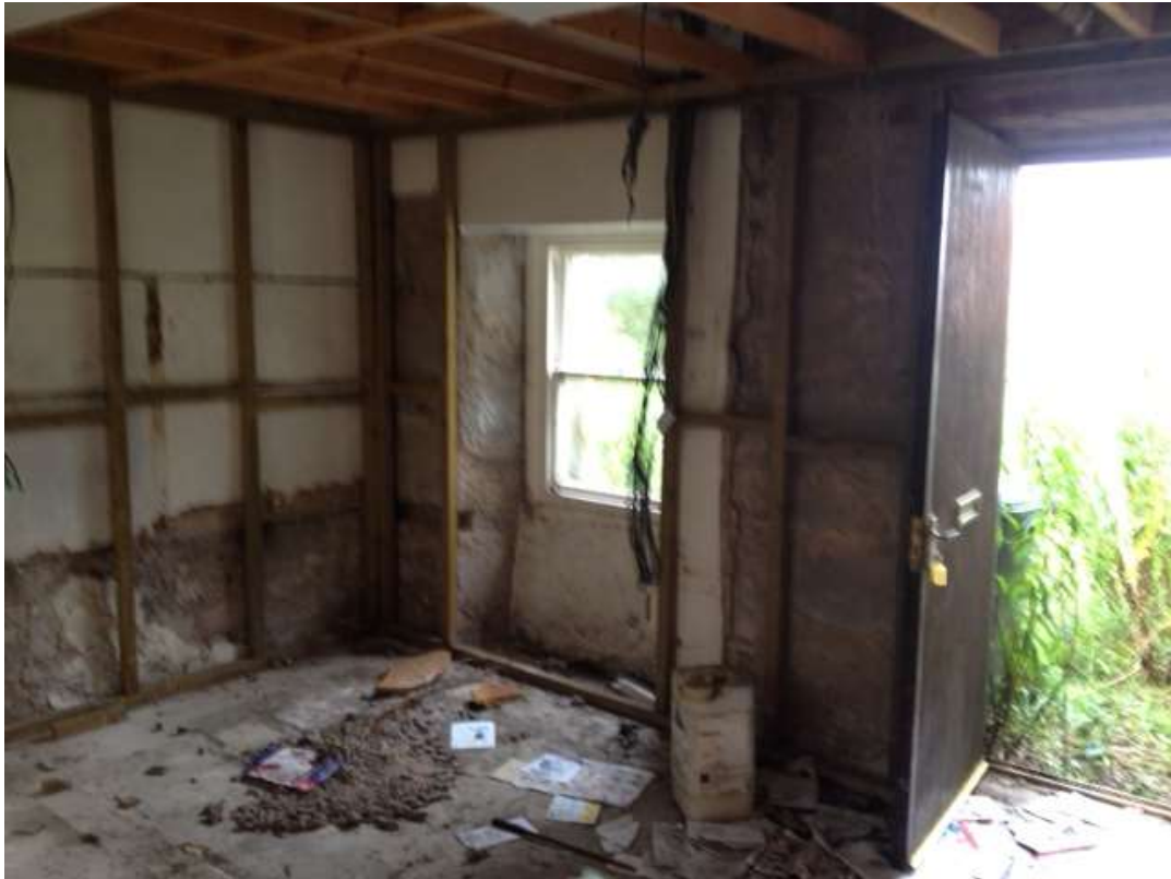
Image showing the decaying interior of the building
