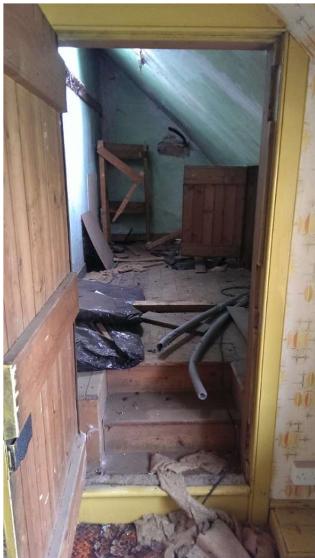
Deteriorating internal image
