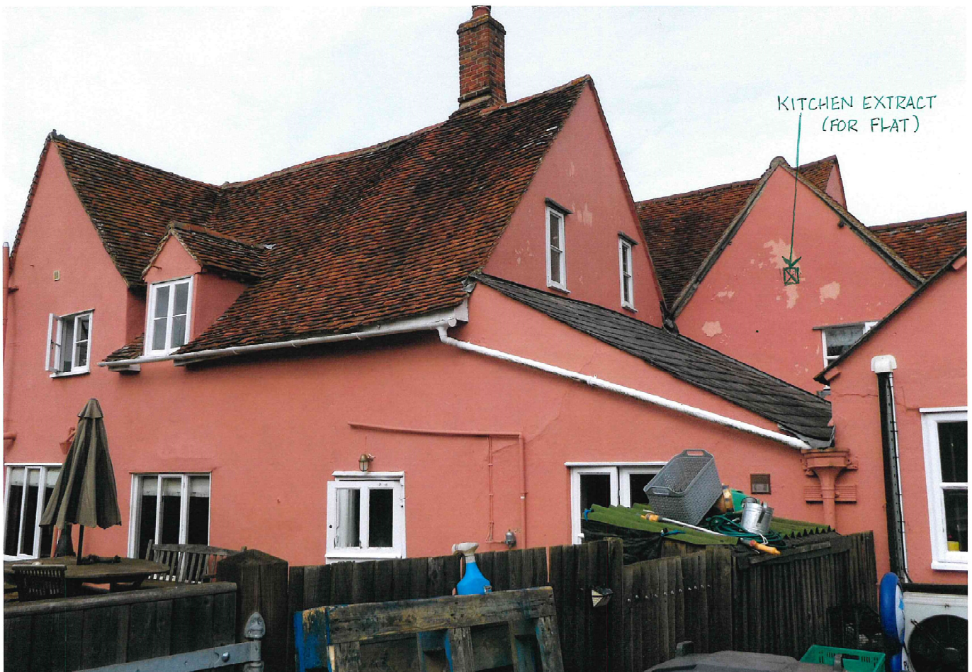
Kitchen (to flat) extract lead covered vent as seen from the rear elevation
