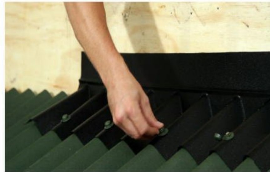
Onduline apron fixing Use Onduline pre-formed apron flashing piece to seal end wall abutments. Lay the upstand against the wall and fix the front apron at each corrugation.
