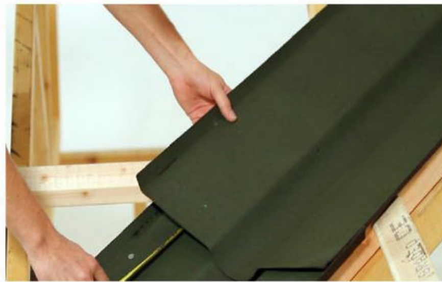
Onduline valley lining Another option is to use pre-formed Onduline valley lining pieces, these laid on fully supporting plywood valley boards positioned.
