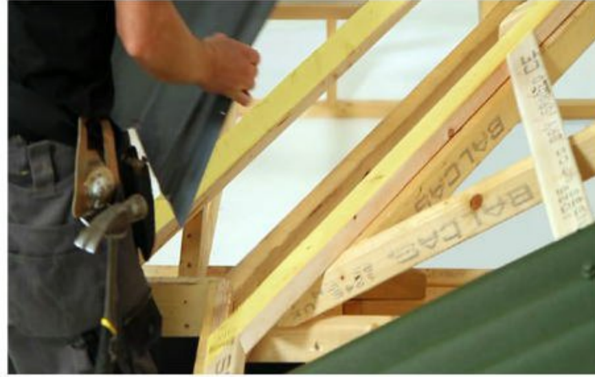
Valley support structure The support structure to the valley is constructed by first fixing trimming battens to the purlins, and lining with valley boards to provide a 7.5cm gutter depth.
