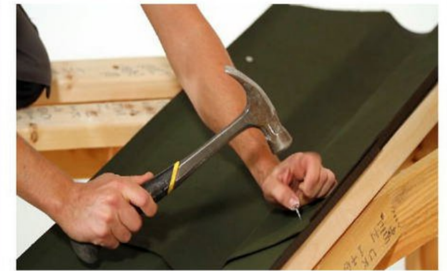
Fixing valley lining The Onduline units are secured to the purlin trimming battens by nailings at 20cm centres up the line of the gutter.
