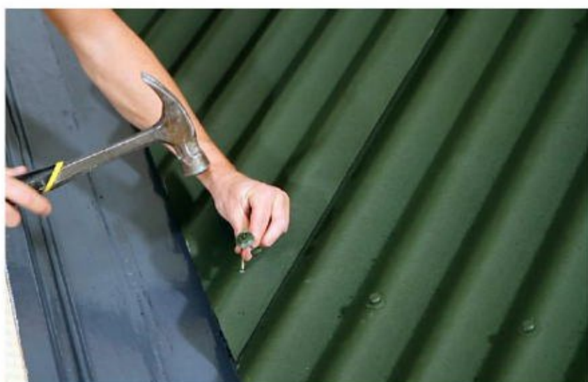
Fixing sheet to valley The sheets are fixed in place allowing for the correct sheet side and end laps. The fixings are secured up the line of the purlin trimming battens.
