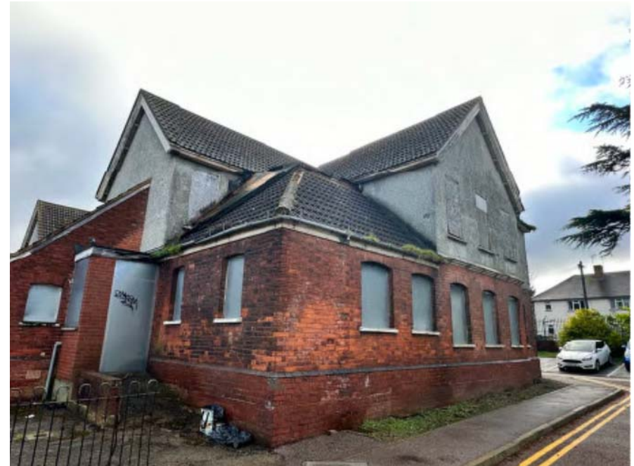
Figure 3- An example of the current condition of the Shamrock Building.
