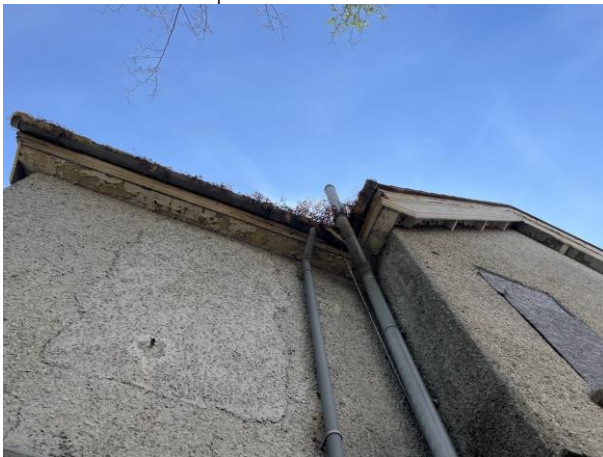
Example of gaps at gable end overhangs at B1
