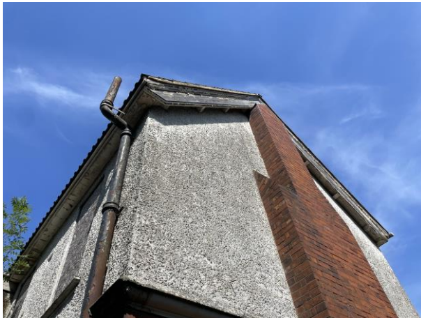
Example of gaps at gable end overhangs at B2
