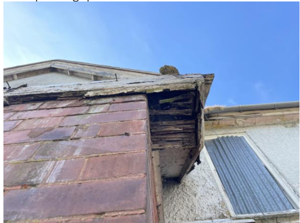
Example of damaged soffit at B2
