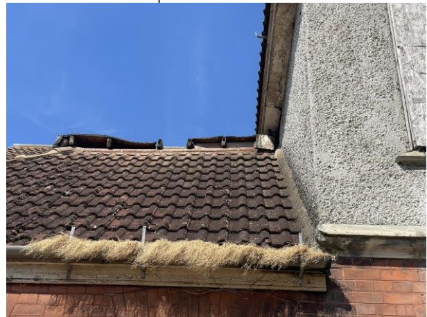
Example of gaps at repaired sections of the roof at B1
