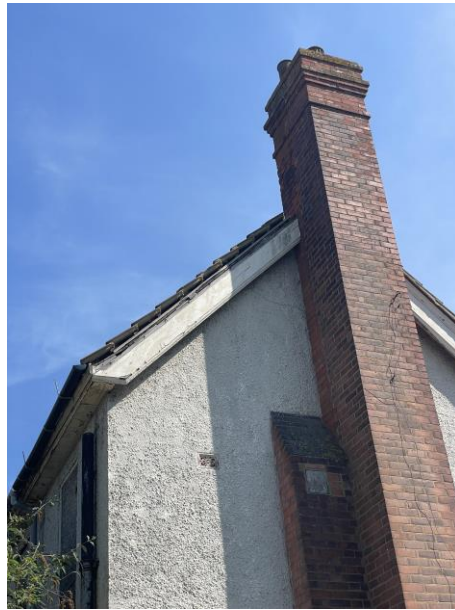
Example of gaps beneath roof tiles at B1
