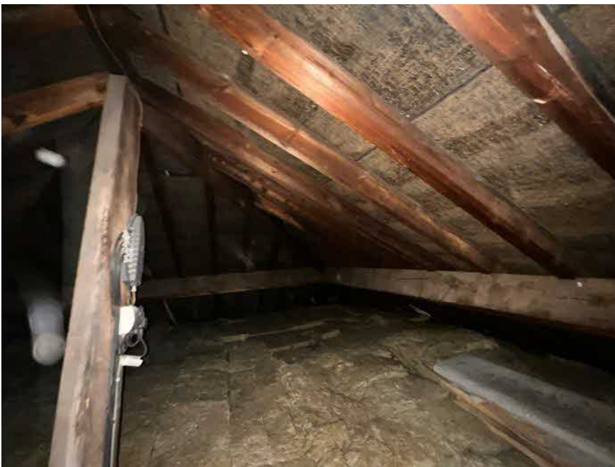
Plate 8: Black lining and insulation in the loft
