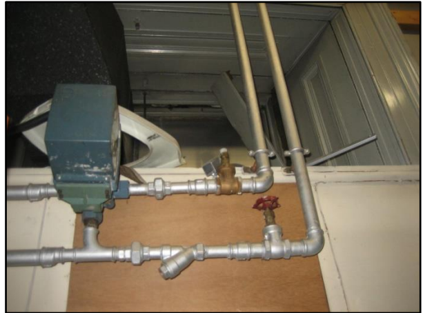
Services in front of boarded over ground floor window
