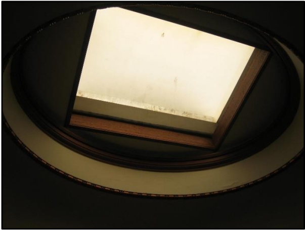
Over stair cupola with dated obscure skylight (to be replaced).
