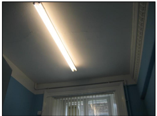
First floor office showing missing cornice/ services penetration
