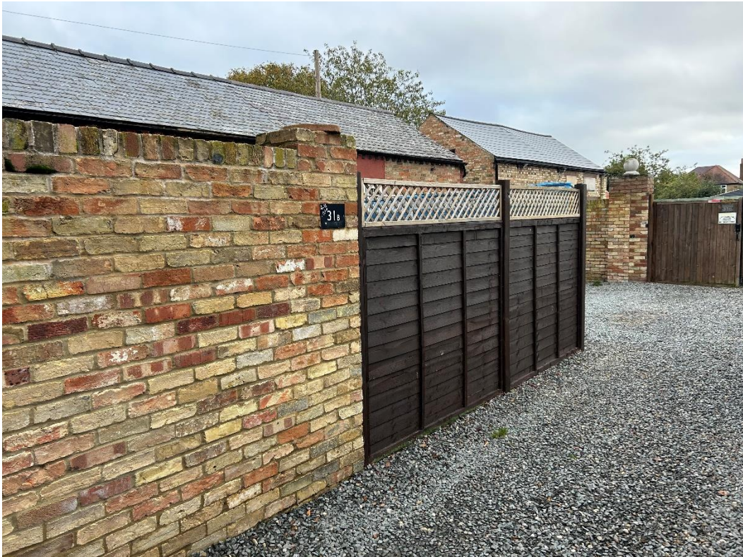
Existing view of boundary wall and fence treatment to the rear of 31b London Road.
