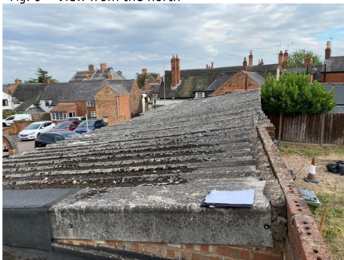
Fig. 9 View from the north showing roof of skittle alley building covered with fibre cement corrugated roof sheeting.
