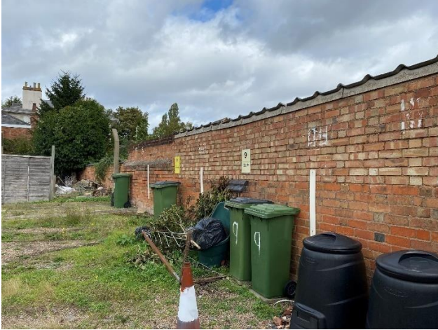
Fig. 10 Western elevation showing side of skittle alley building built up above an earlier brick wall.
