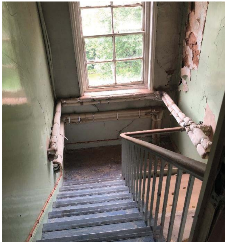
Figure 42: Blocked stairwell within the building
