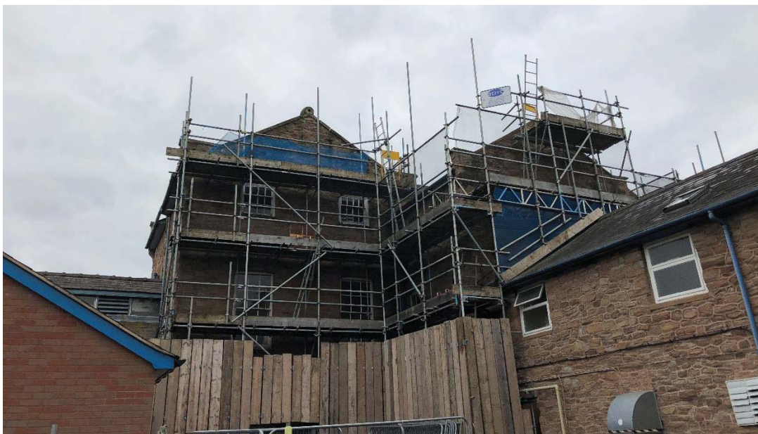
Figure 19: Rear view of the upper floors of the entrance block to the south (scaffolded).
