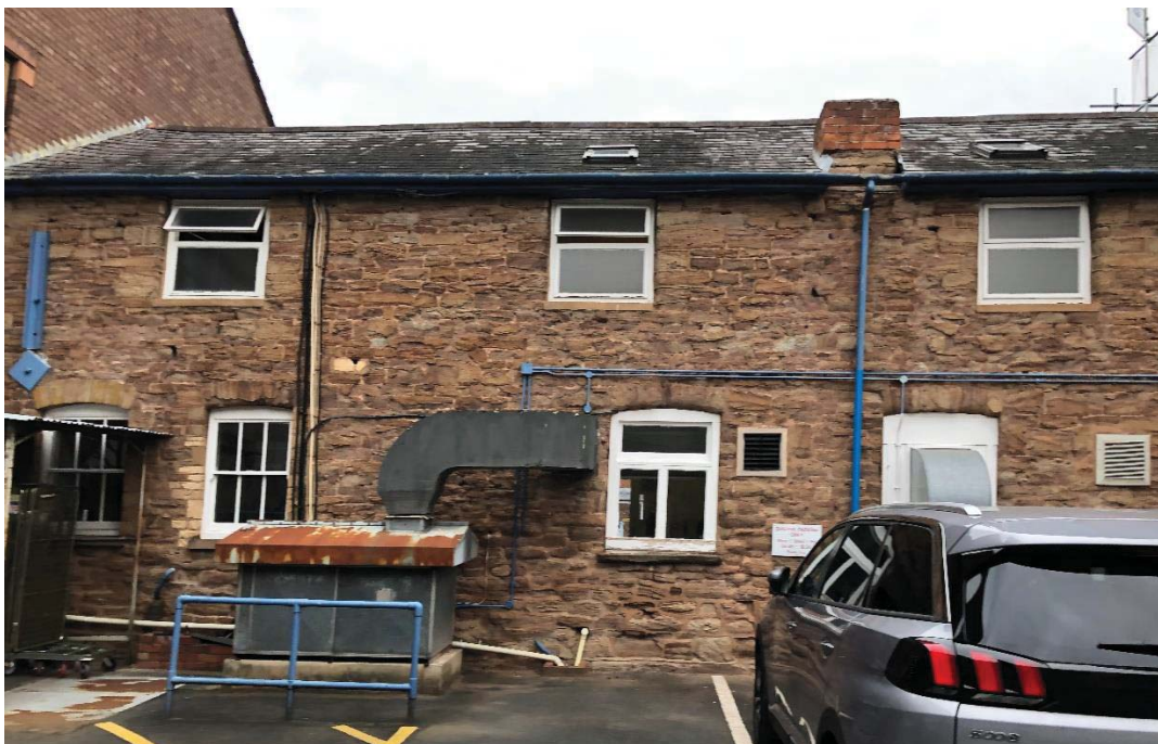
Figure 17: Rear range (radial 'spoke') western elevation adjoining the later 20 th century hospital building to its north, and showing brick replacement chimney stack, replacement windows and inserted ventilation and ducting.
