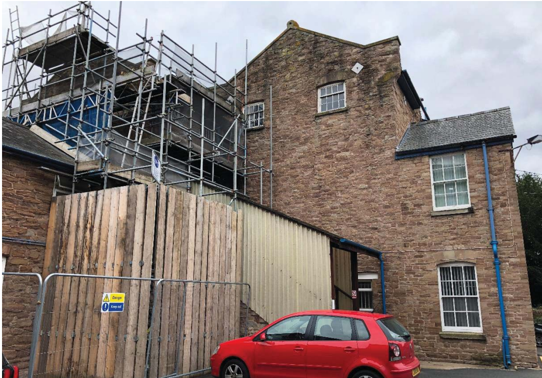
Figure 16: rear elevation of the entrance block showing original fenestration to upper floors, scaffolded and cordoned stairwell to access.
