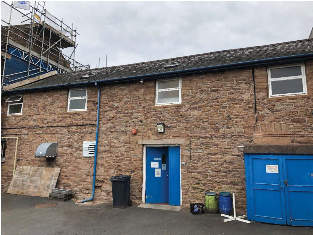
Figure 18: Rear range (radial 'spoke') eastern elevation adjoining the entrance block to the south, hospital building to its north, and showing replacement windows and doorway alteration.
