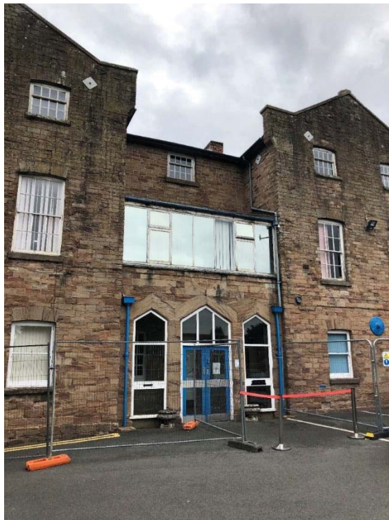
Figure 12: View of the later porch and glazed balcony and original and replacement fenestration
