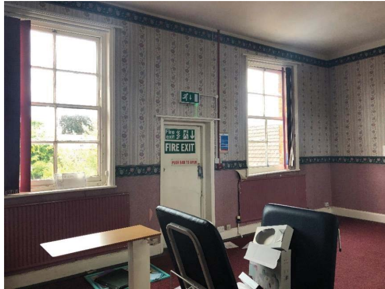
Figure 43: Rear room on first floor, original wooden frame sash windows and modern fire escape
