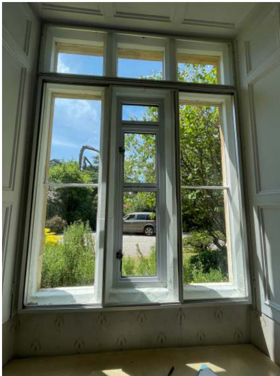
Fig. 12 (Left): Stone mullioned windows to reception rooms with decorative panelling to top reveal and panelled shutters. Windows fitted with secondary glazing and uPVC double glazed opening lights which detract from the aesthetic and architectural significance of the building.
