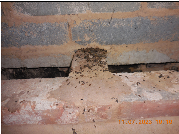
Plate 8. Concentration of bat droppings at the eastern gable end of Roof 3, adjacent to a chimney cavity
