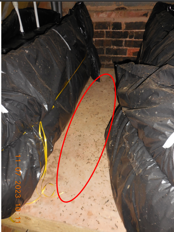
Plate 6. Scattered bat droppings (red circle) under the ridge within Roof 2
