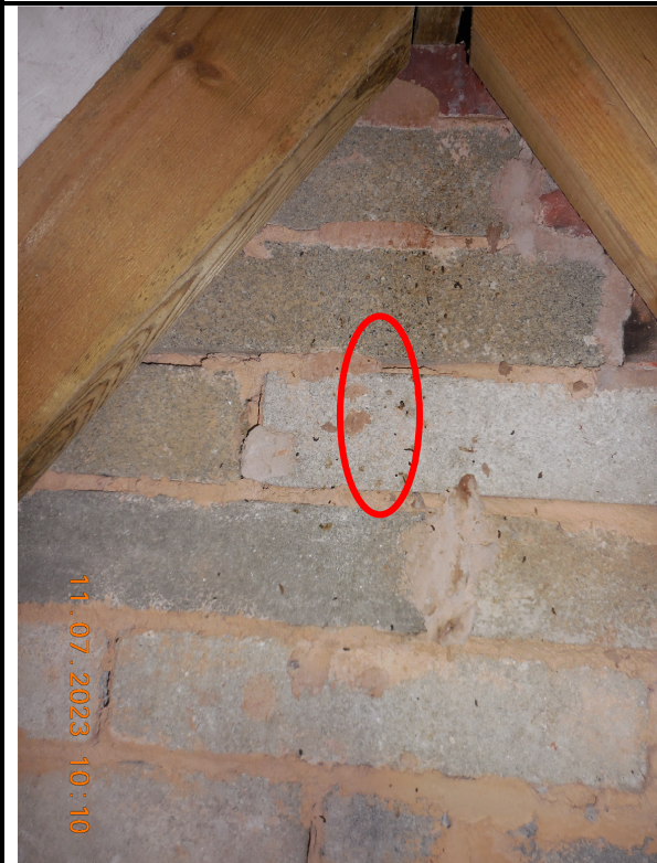
Plate 5. Bat droppings on the internal gable wall within Roof 2 (red circle)
