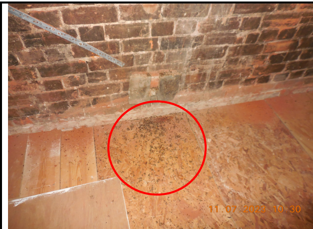
Plate 7. A concentration of bat droppings (red circle) within Roof 2
