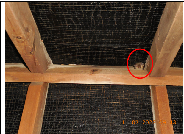
Plate 5. Brown long-eared bat (red circle) seen roosting in Roof 1
