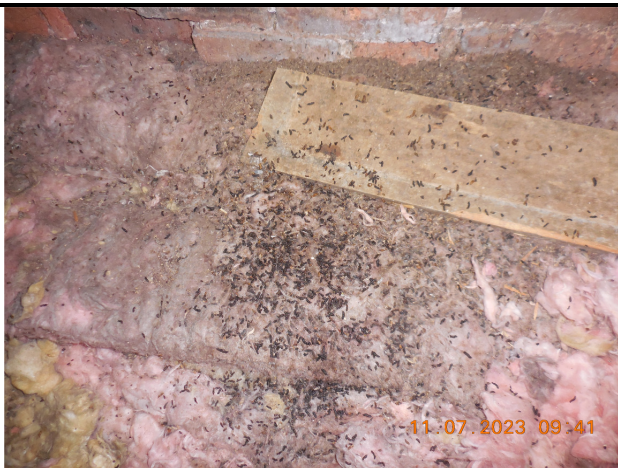
Plate 6. Concentration of bat droppings at the southern end of Roof 1
