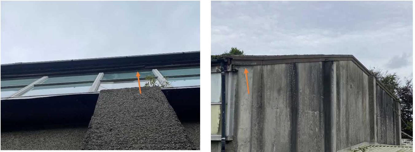
Figure 11: Low numbers of gaps were present on the gable end and southern side of the assembly hall.
