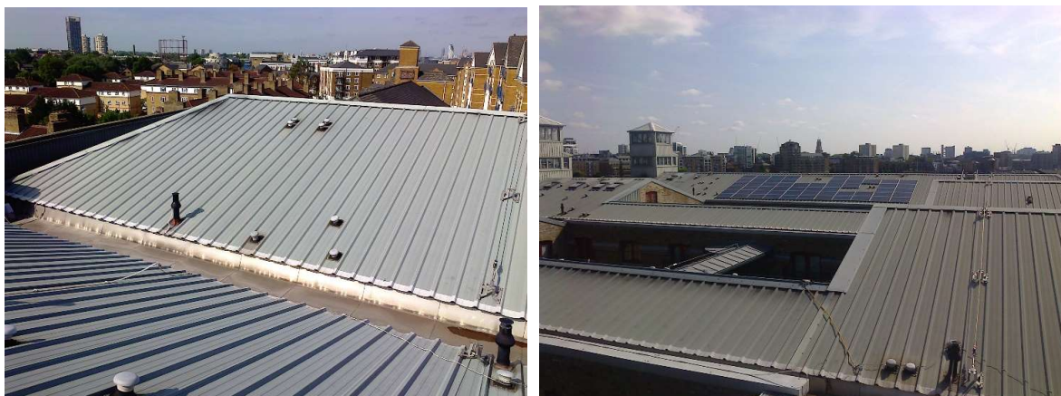
Image 7 (above left) shows the roof above Flat 113 Globe Wharf, looking south, and shows the buildings perimeter wall (top left) that conceals sight of the roof from the street and neighbouring developments including Lavender House opposite. Image 8 (above right) shows the view looking eastwards from the roof of Flat 113, showing solar panels installed on one of the west-facing roof pitches and other skylights installed in the roof (e.g. top left).
