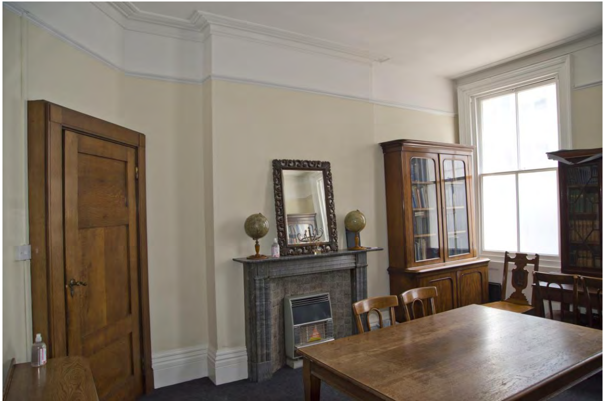
Plate 41 – No. 25 Queen’s Road, northern ground floor reception room, original fireplace. Note Phase 3 inserted door. View looking north-east.
