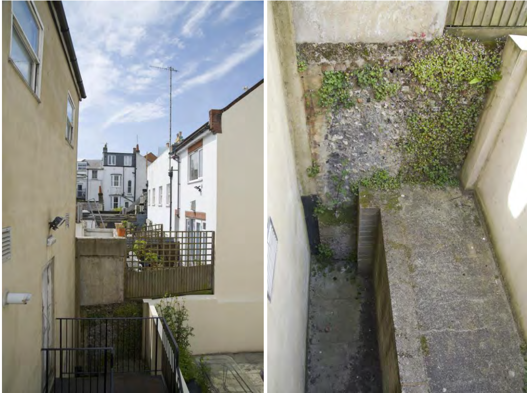
Rear lightwell to No. 24. Note the original garden wall in this area
