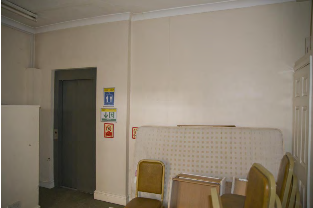
Rear wall of Phase 1 house at first floor level, where a new doorway is proposed to be inserted.
