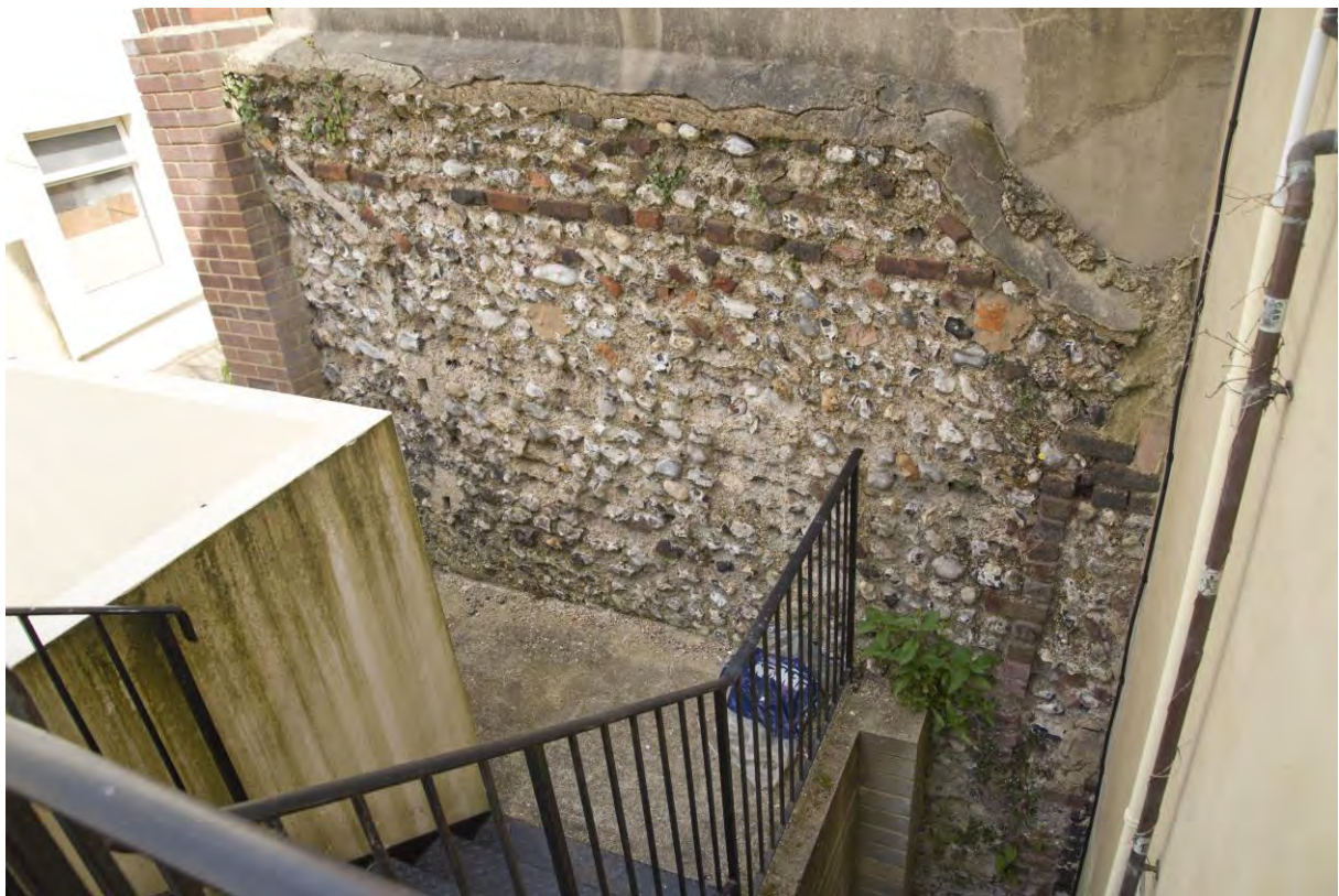
Plate 37 – Phase 1 bungarosh garden wall to the rear of No. 24. View looking north.
