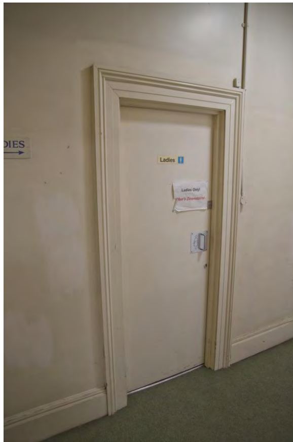
Plate 39 – No. 25, original architrave to suspected Phase 1 first floor service passage. View looking south-east.
