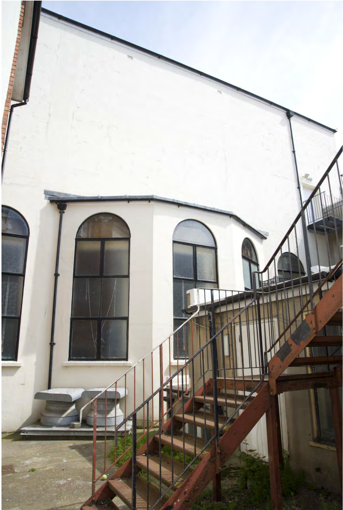
Plate 58 – No. 25 Queen's Road, side elevation to Phase 3 northern extension. View looking north.
