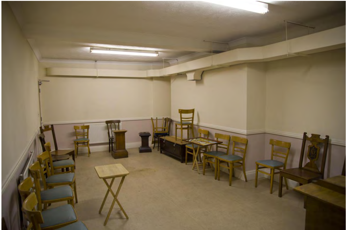
Plate 27 – No. 24 Queen's Road, rear cellar room (suspected original kitchen). View looking east.
