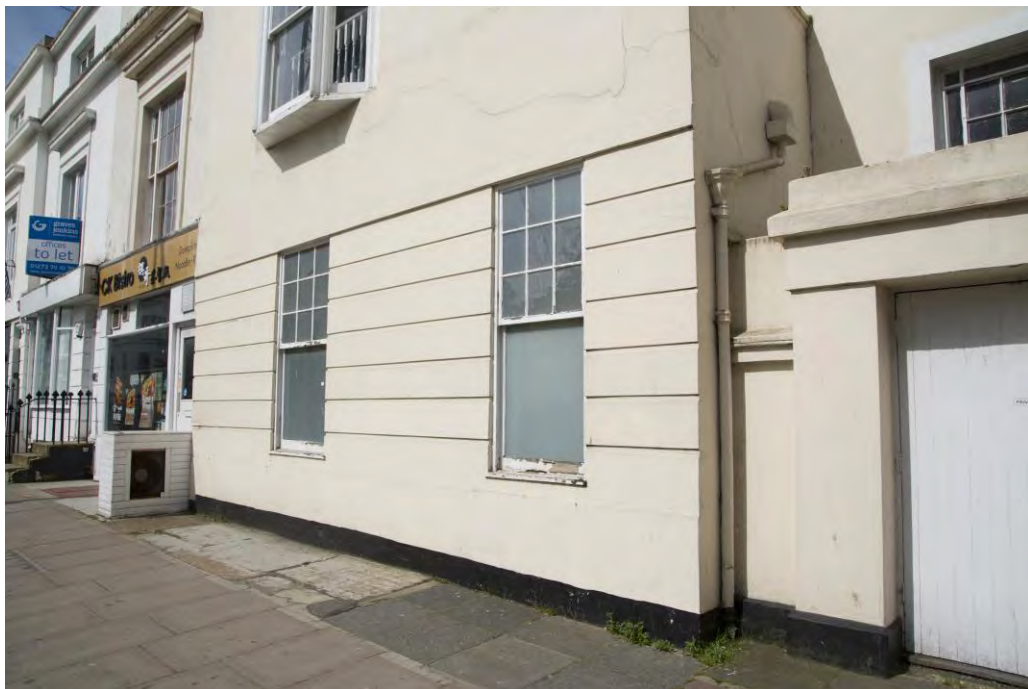
Street frontage of No. 24, showing the blocked former lightwell.
