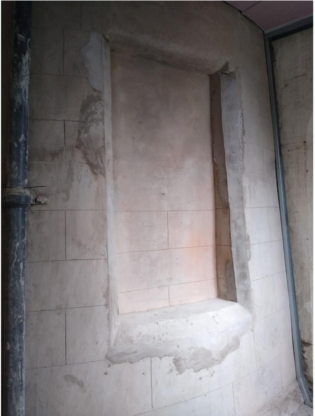
View of Existing Cement Render
