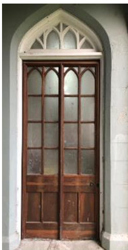
View of Original Door and Fanlight (in storage) to be retained, restored and relocated.
