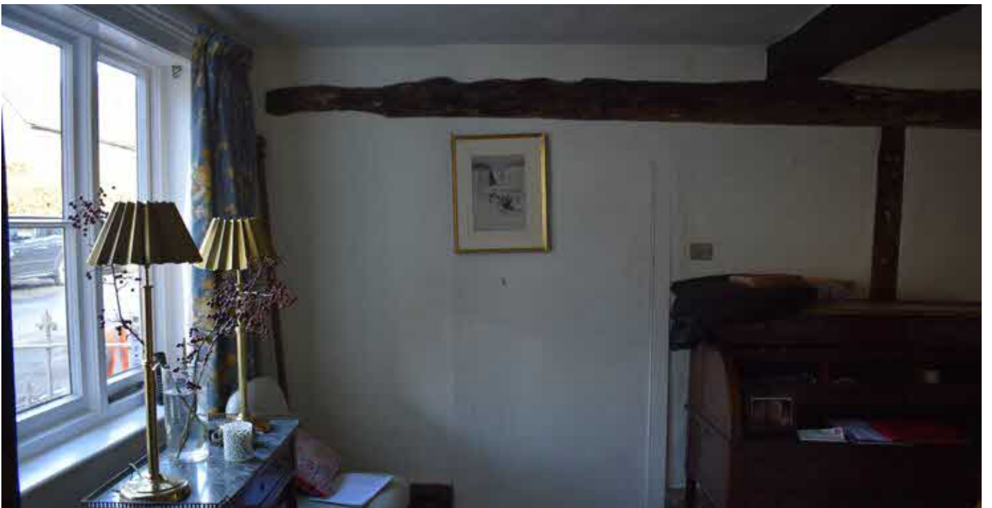
Infilled doorways connecting to the neighbouring house, consistent with the information on the tithe map of 1850 which shows both buildings in the same ownership.
