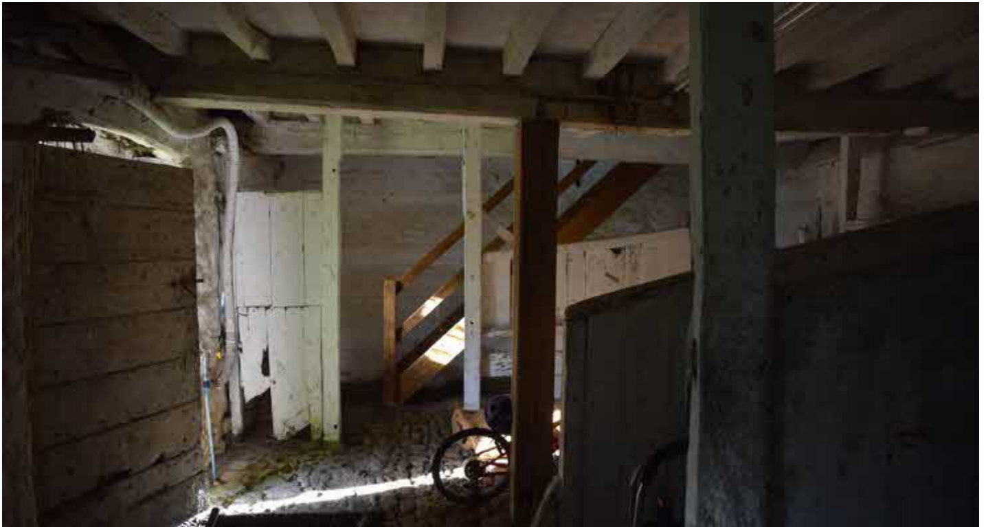
Ground floor stables with Irregular stone cobbled floor and timber framing supporting upper floor.
