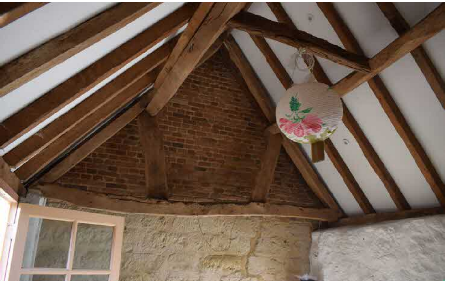
Interior of studio room has stone wall where abutting stable, with brick above eaves level. Exposed roof trusses and stone floor.
