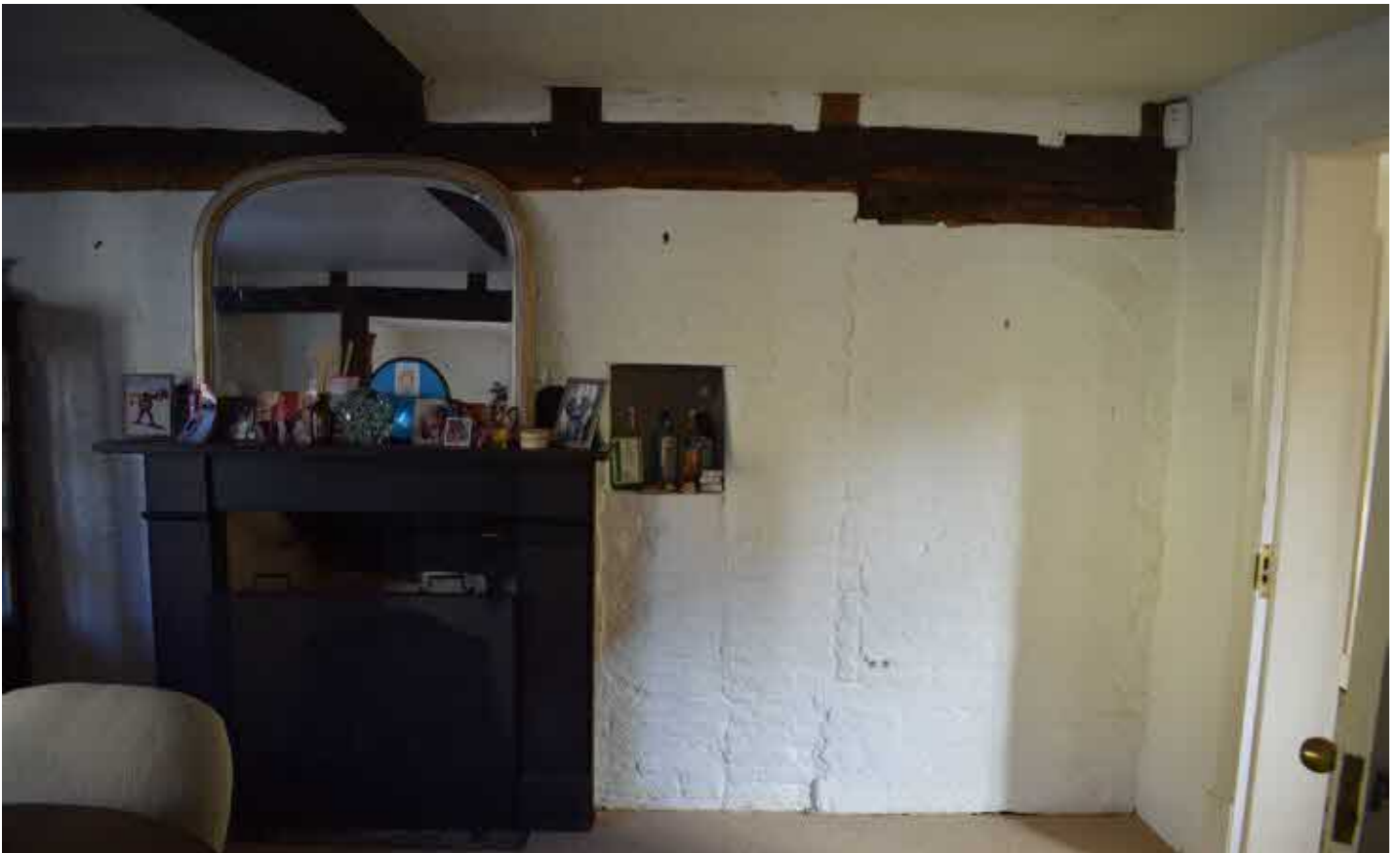
The main Sitting room fireplace now has a modern surround, however the brickwork niche and arch adjacent appear to be of an earlier date.
