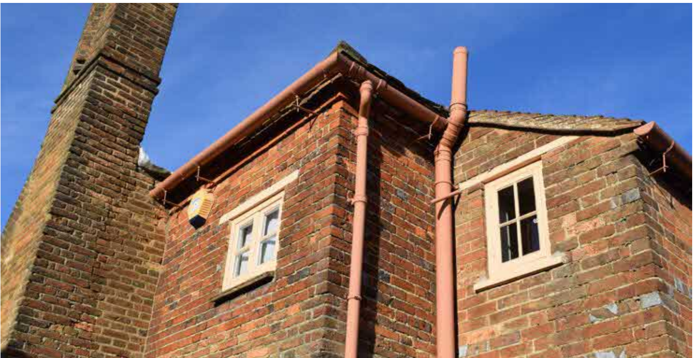
Detail of south elevation showing phased construction of chimneystack and rear corridor
