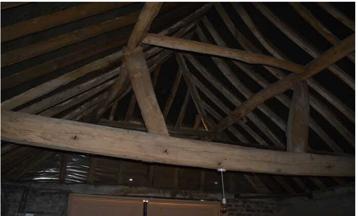
Garage - exposed painted brick walls to three sides, with stone rubble wall to perimeter boundary (just visible). Timber queen post or strut to roof truss, purlins and rafters exposed. Quality and detail of framing suggests 18th century date.
