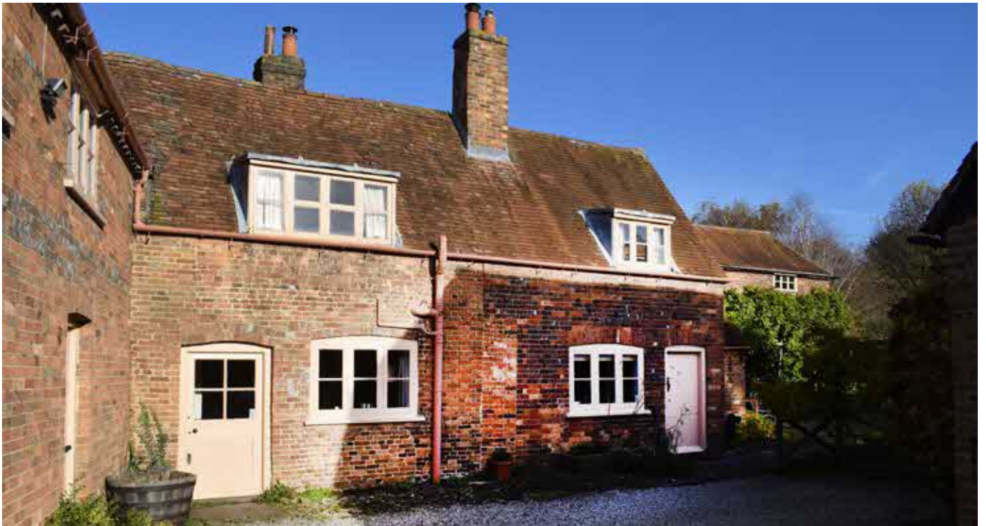
Ancillary rear range with straight joint and two brick types indicating two phases
