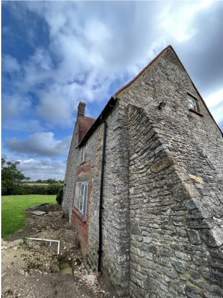
Huge Buttress tilting away from building. Excavations also laying with water.
