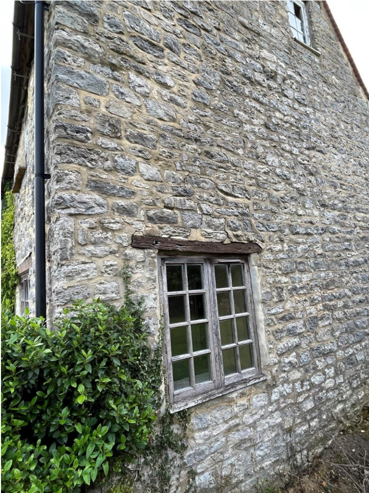
Lintel failure to lounge window.
