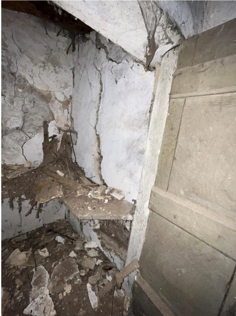
Cracking in bedroom cupboard to Western elevation (adjacent to southern gable)
