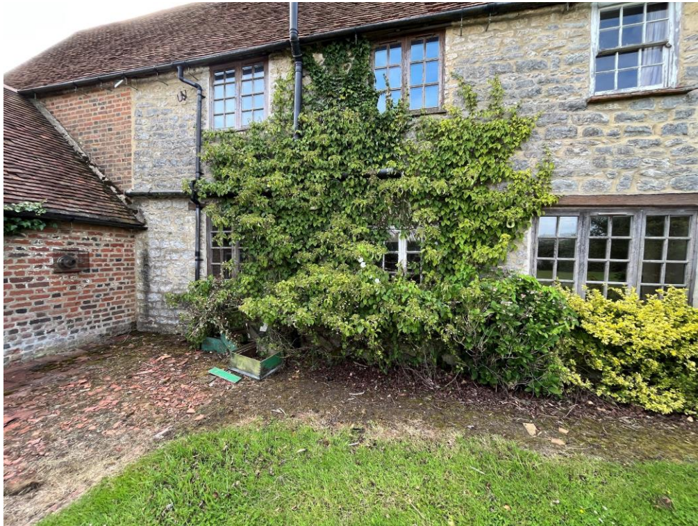
Large creeper/climber covering windows. Holding moisture against the building
