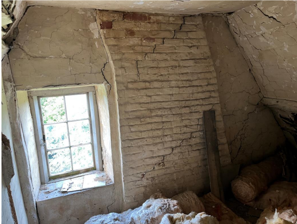
Tension cracks to masonry, Western Gable
