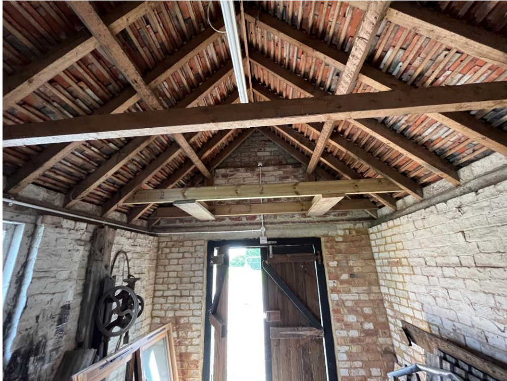
Storeroom with some additional ties and props to purlin bearings.
