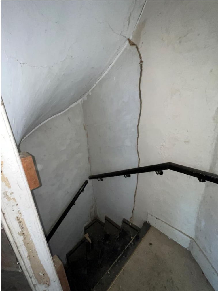
Vertical crack, ground to first floor stairwell (adjacent to southern gable)
