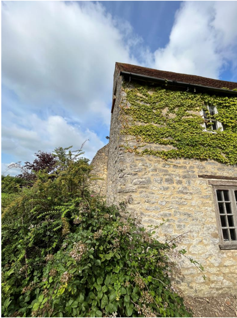
Southern Gable end, verge leaning outwards allowing water into the wall.
