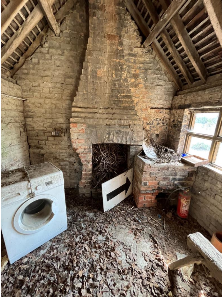
Roof spread to forge, cracking at vertical junctions of walls.
