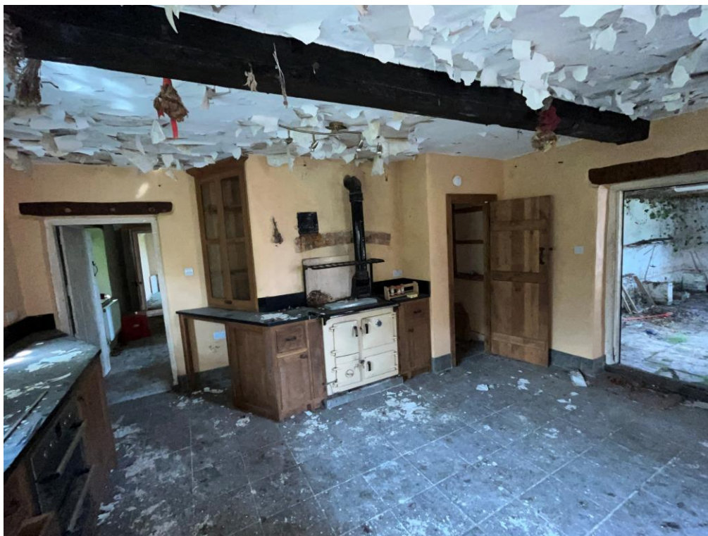
Kitchen, dampness behind range, ceiling paint peeling.
