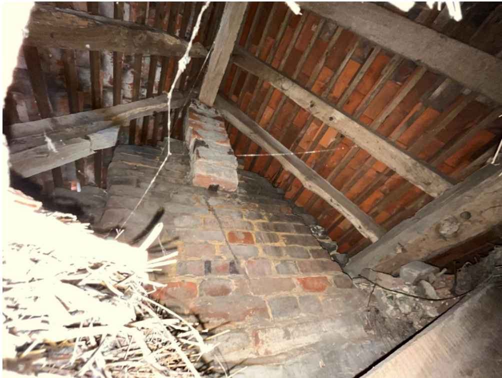
Southern Gable in 2 storey section. Corbelled brickwork propping ridge.
