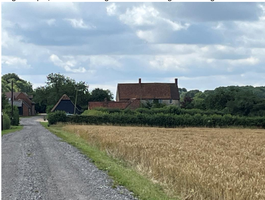
Visible tilt to ridgeline from afar. Note downward slope on RHS towards Western chimney/gable.
