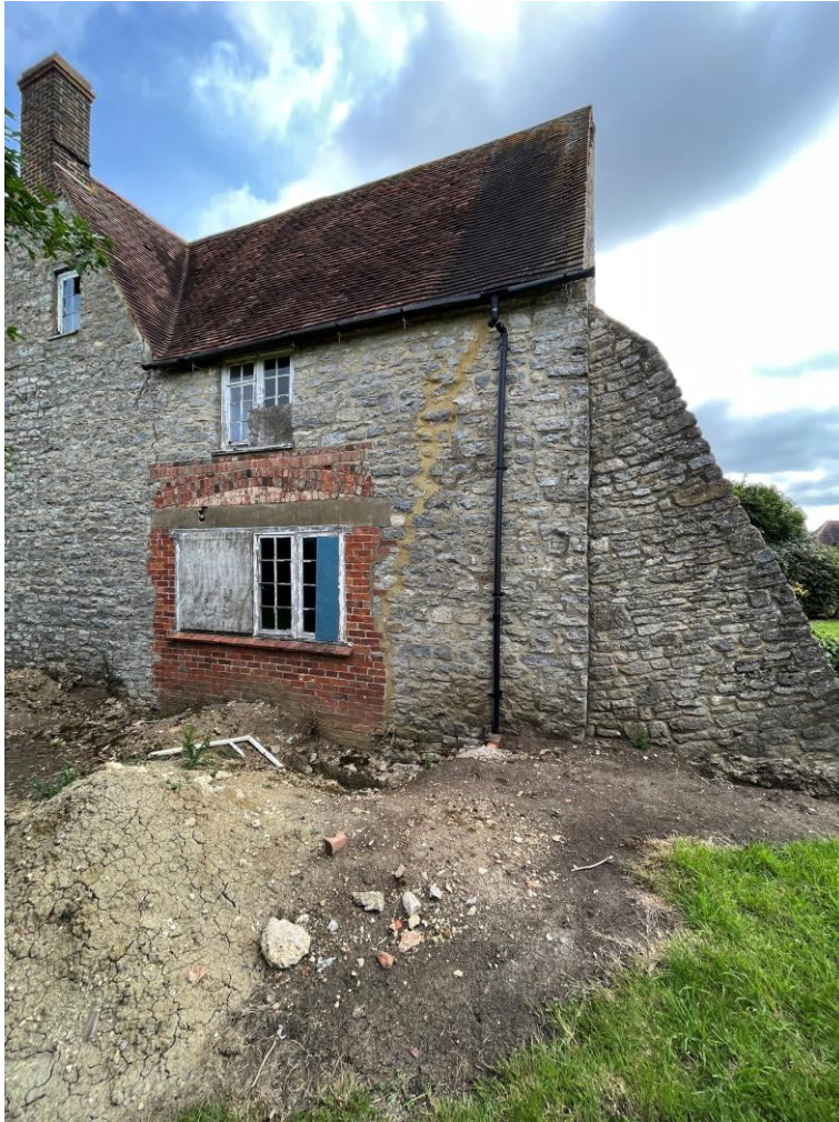
Cracking to Western elevation either side of masonry panel. Disconnected downpipe, Modern machine-made tiles near verge end.
