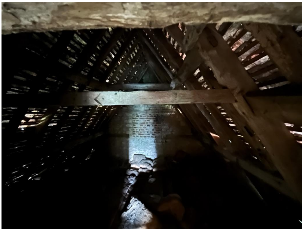
Holes in tiling in roof space.
