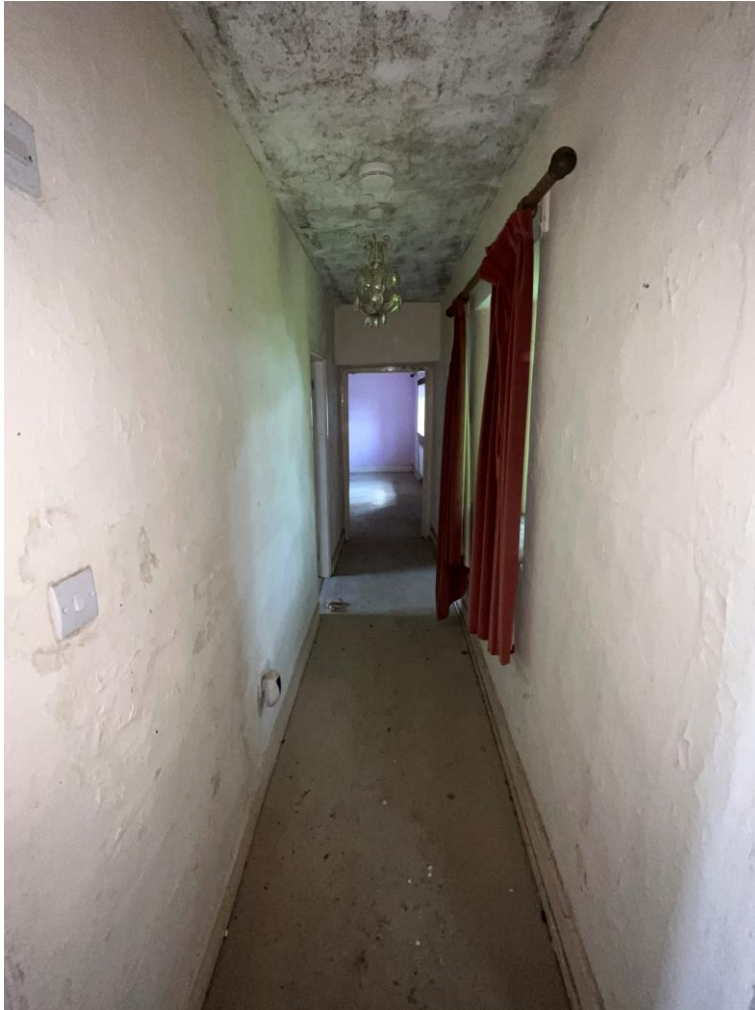
This photo doesn't show it clearly. But Main bedroom door out of Square, floors and door heads sloping. Also, walking uphill towards door.
