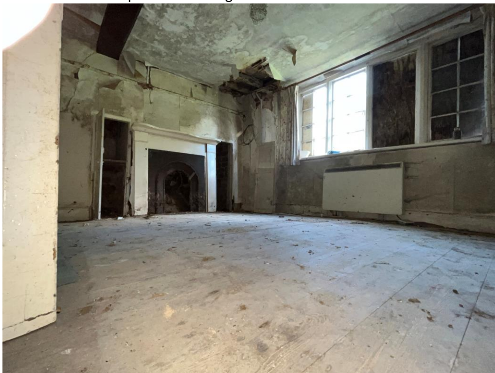
Floor bulging and dipping to Western elevation.
