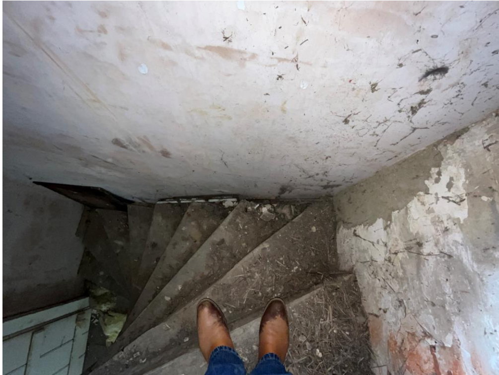
Gap between string and wall, Southern gable
