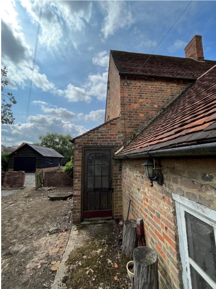
Missing lead flashing to porch, and poor condition of mortar fillet at abutment.
