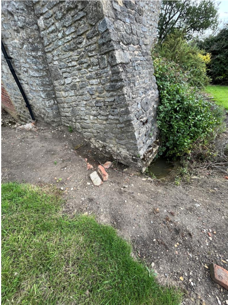
Water laying around undermined buttress.
