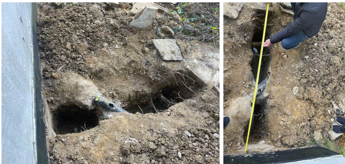
Photograph 3 and 4: showing the location and sizes of the most substantial roots encountered.
