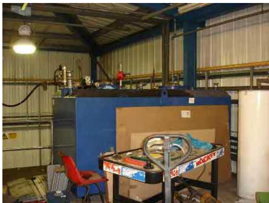
PLATE 5: Evidence of hydrocarbon spills at Unit B.
