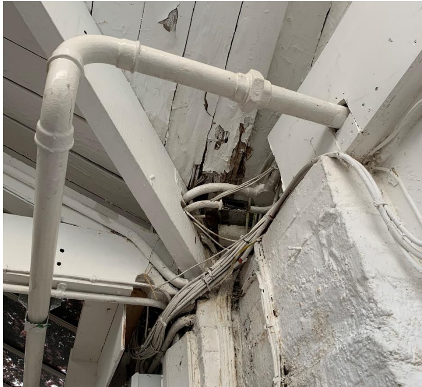
Figure 5 - Evidence of water ingress (Survey Photo)
