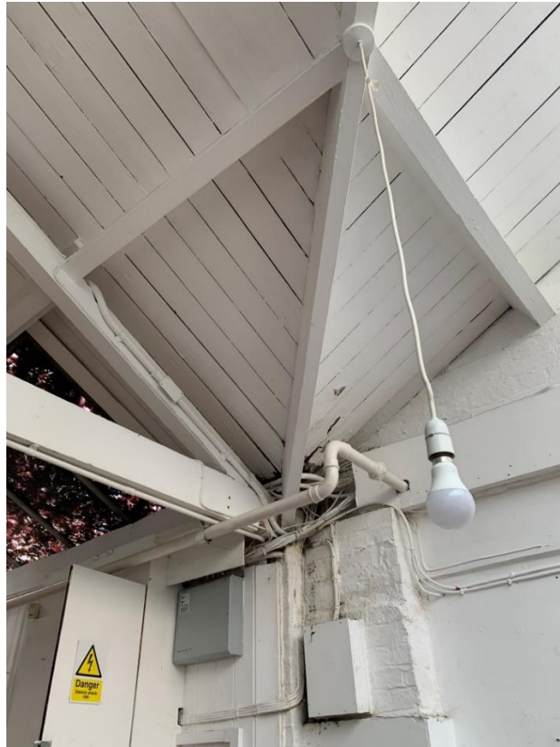
G.RM 07 – ROOM 3: Wall & ceiling finish to be repaired.
