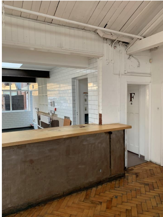
G.RM 06 – ROOM 2: Rotting roof structure to be repaired.
