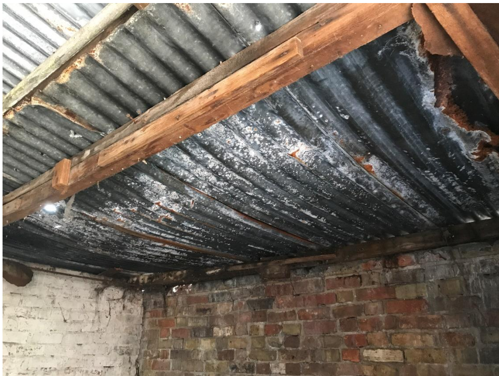
Photo 28 – Outbuilding, underside of west roof.
