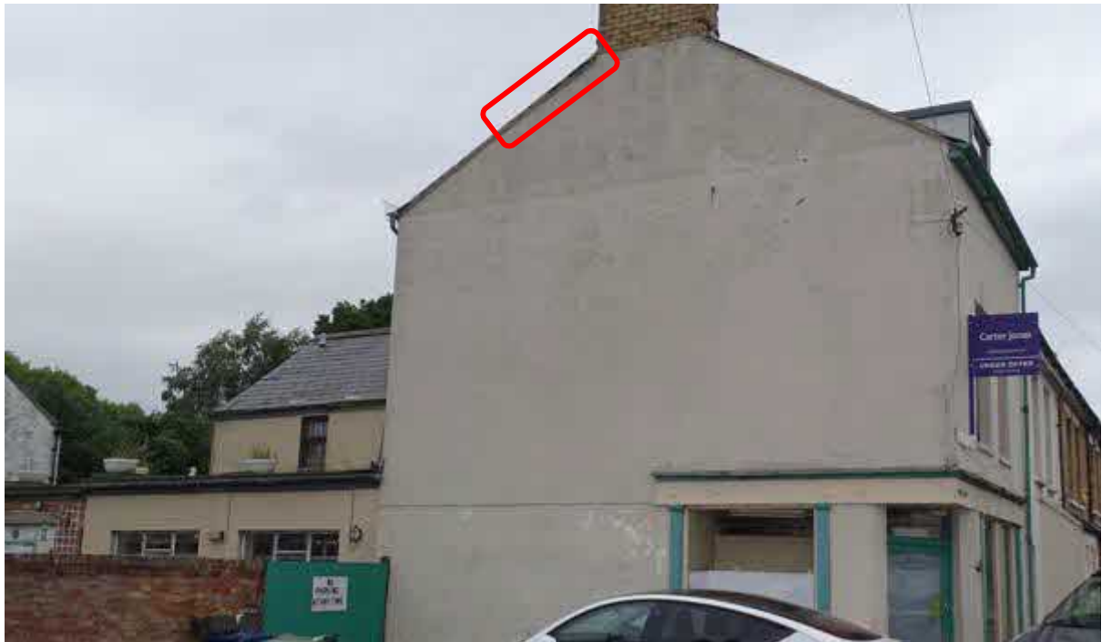
Image 3 – West facing elevation of the three storey section where gaps between the roof coverings and stonework's below look to provide further opportunities for bats
