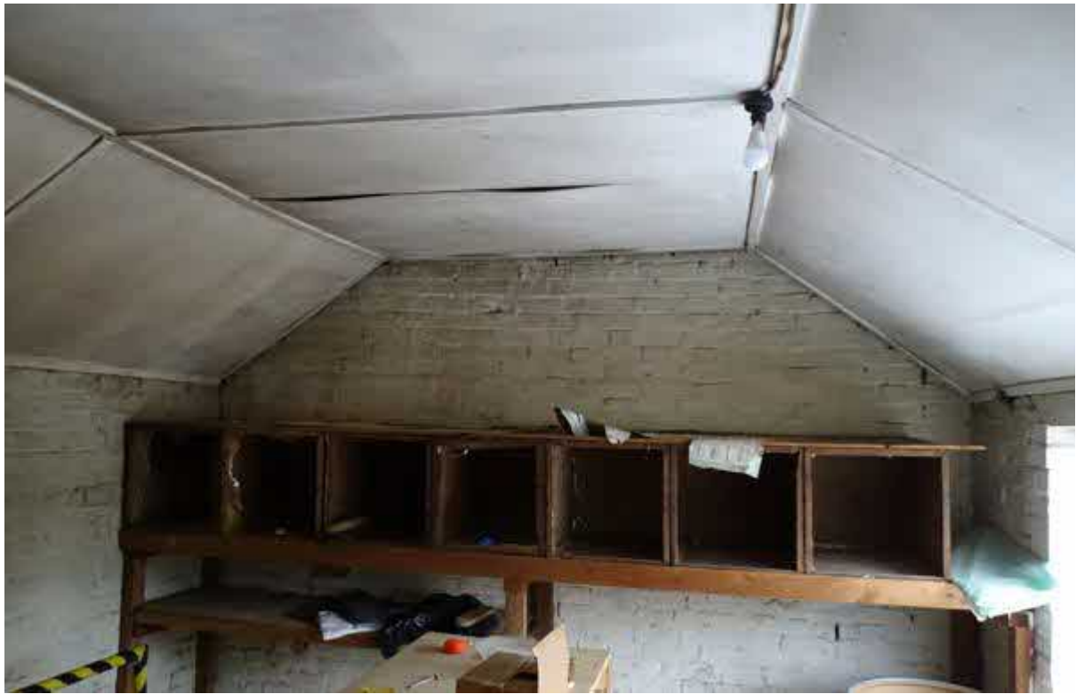
Image 11 – Internal view from below the roof areas as per image nine on the previous page
