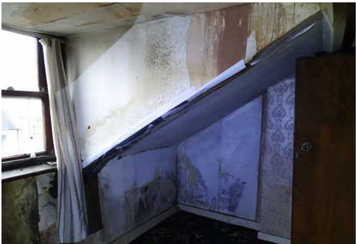
Image 6 – Internal view from within the three storey section of the building where no accessible roof void spaces are provided
