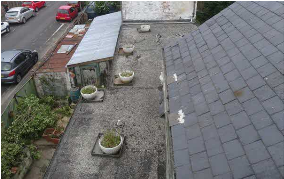
Image 7 – View across the flat roof areas of the mid section of the site
