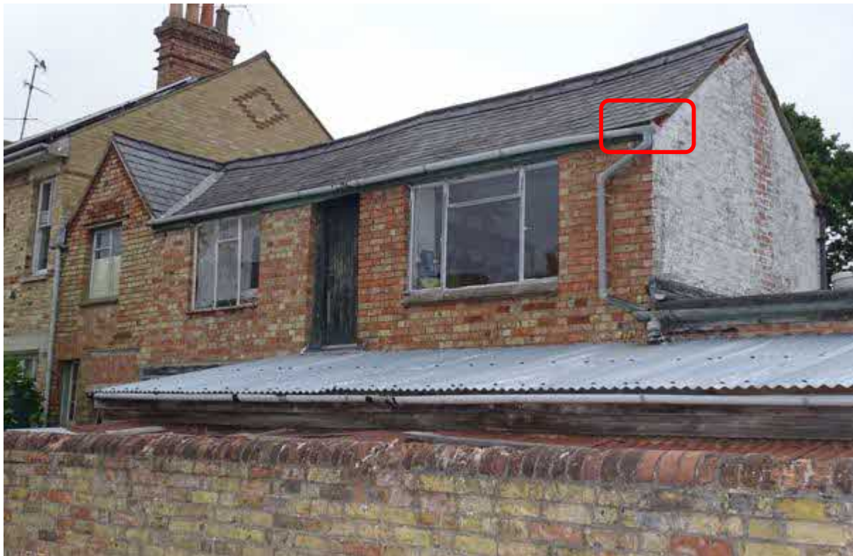
Image 9 – West facing elevation of the two storey structure to the far North of the site where gaps between the roof coverings and brickworks look to provide further shelter/access opportunities for bats
