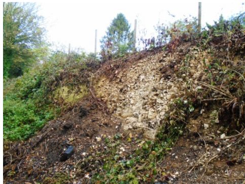
Figure 8 View of part of the chalk face on the north eastern side of the cutting.
