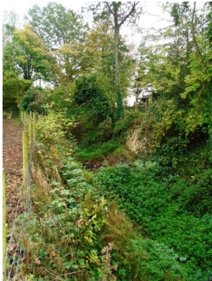
Figure 10 View looking southwards from the north-east side of the cutting; note the fragment of the chalk face.
