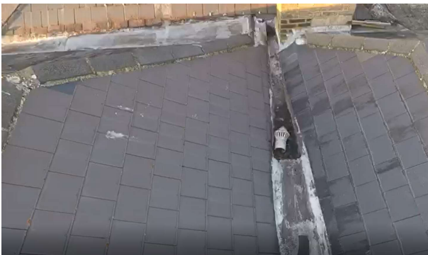
Valley gutter to internal outlet and valley gutter for altered gutter to fall to beyond.
