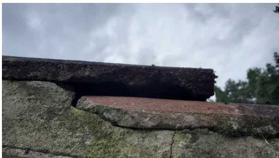
5 gap under tile on north gable (confirmed roost)
