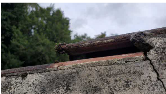
7 gap under tile on south gable (possible access)
