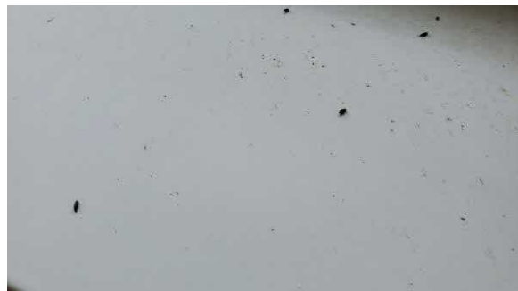
6 bat droppings under roost access
