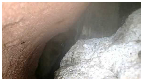
8 bat under roof tile. Poor image due to light reflecting from cement closer to the endoscope
