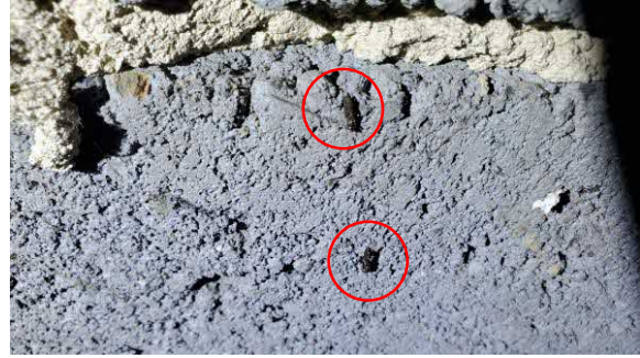
10 bat droppings on internal gable wall
