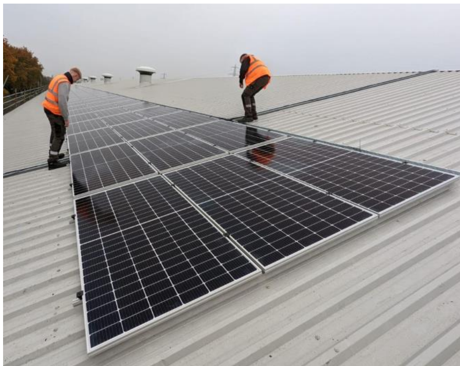
120kWp roof mounted solar PV installation on a poultry house completed by NerG Ltd
