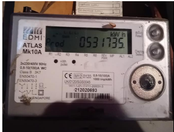
Typical PV generation meter.
