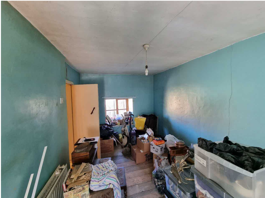
Photograph No. 12 – View On To Rear Wall Of First Floor Right Hand Bedroom
