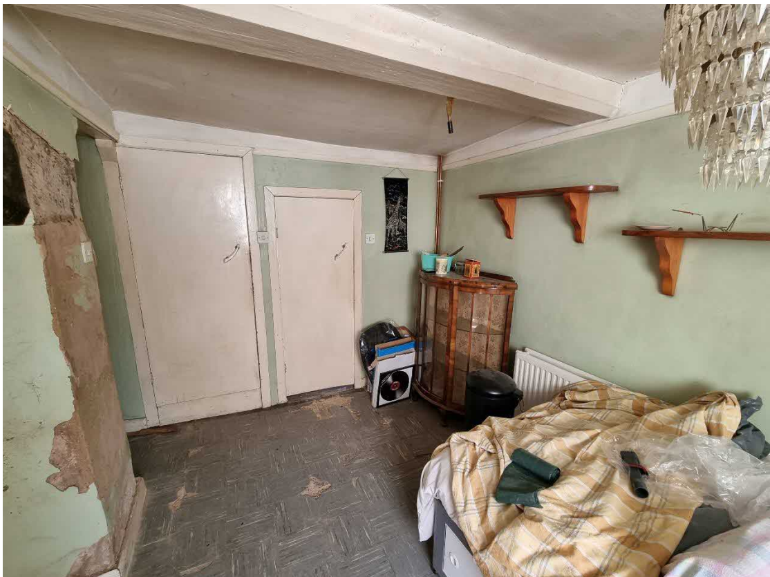
Photograph No. 10 – View On To Ground Floor Right Hand Bedroom Rear Wall
