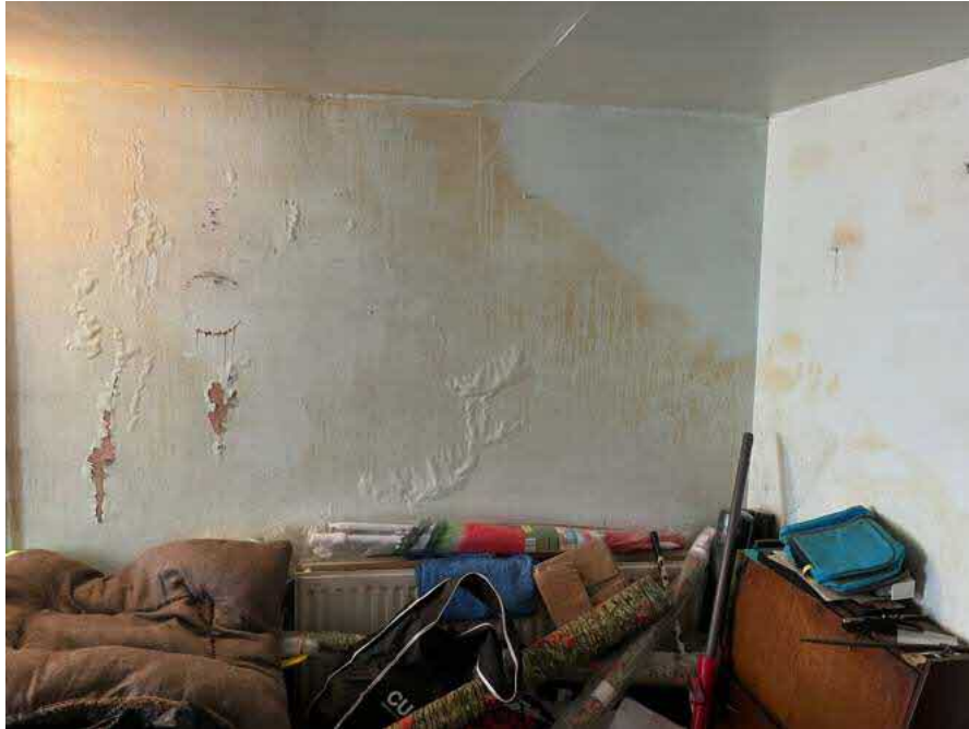
Existing dining room showing damp walls etc.
