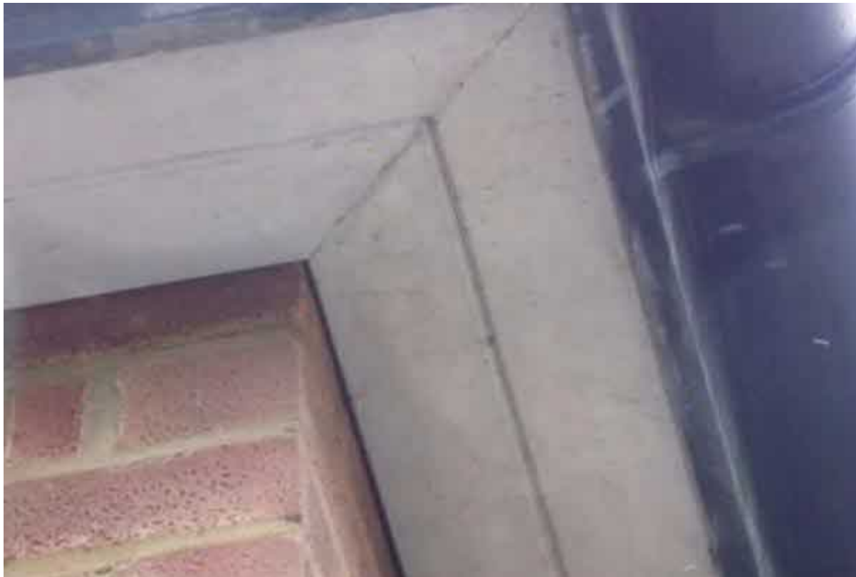
Image 5 – Close view of the main eaves coverings which have demonstrated a fair level of condition throughout
