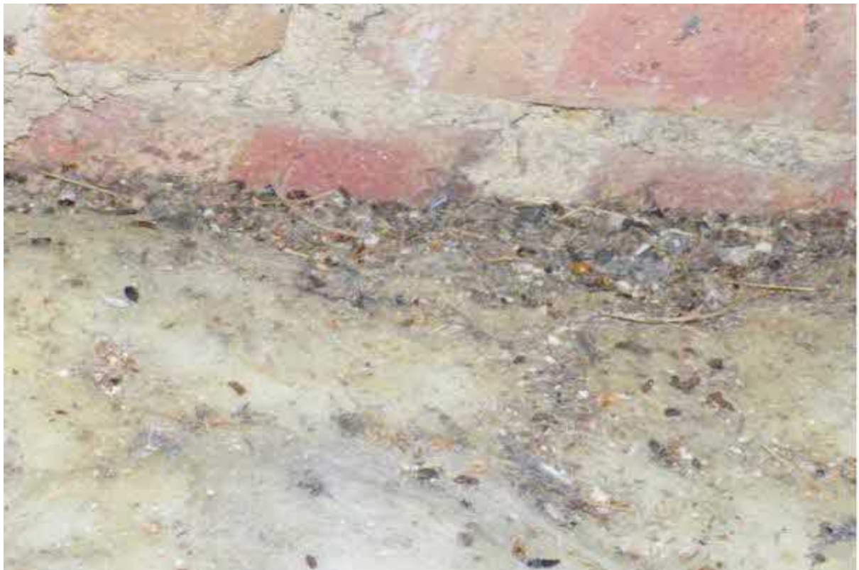
Image 10 – Further images of droppings within the main roof void spaces of the property
