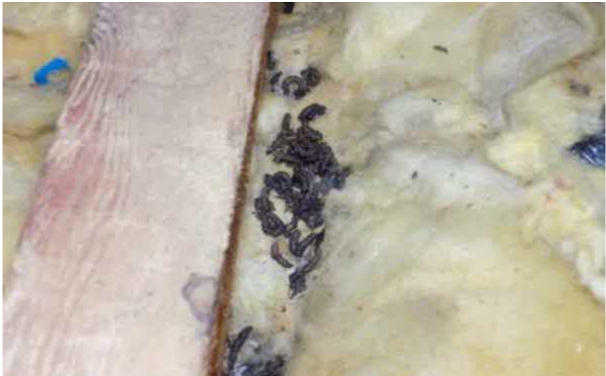
Image 9 – Further images of droppings within the main roof void spaces of the property
