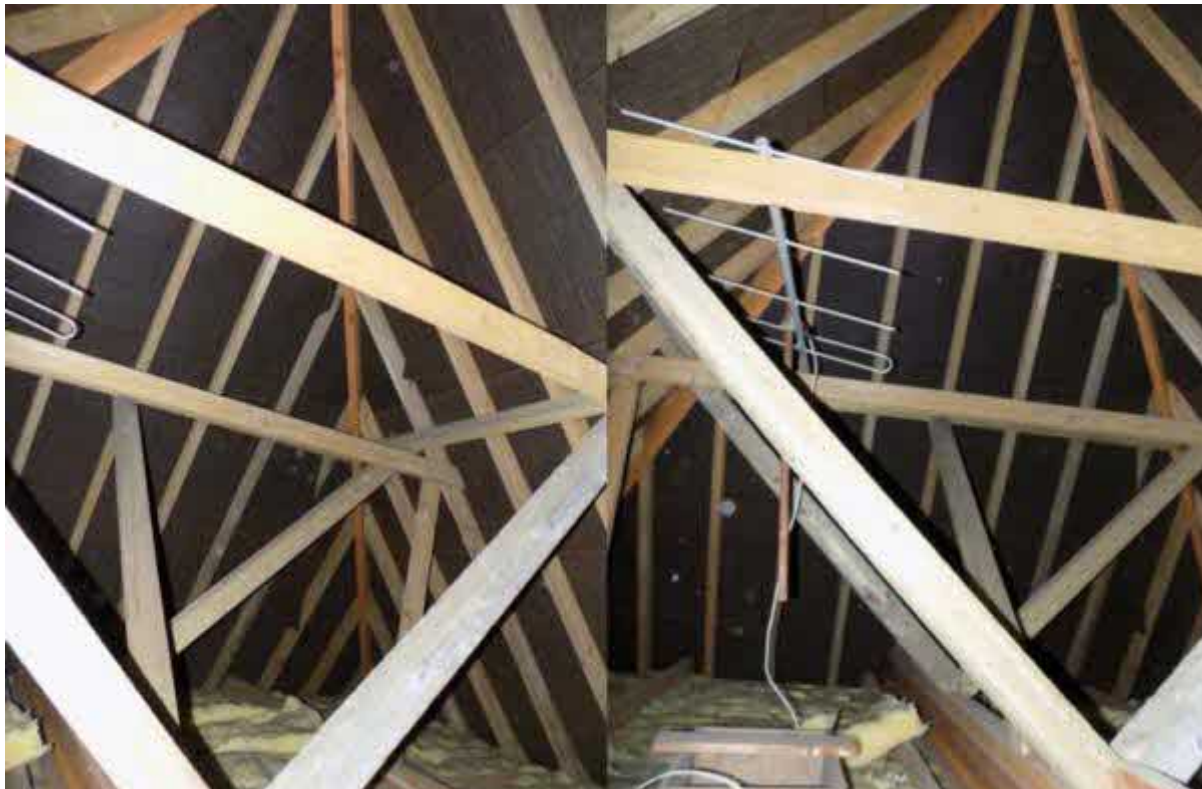
Image 6 – Internal view from within the main roof void spaces of the property
