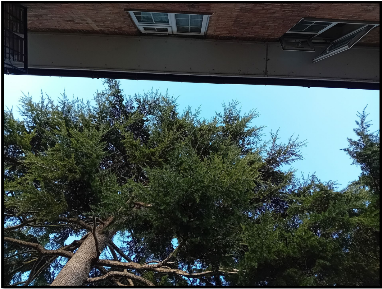
Figure 8: Photograph to demonstrate the current clearance of tree T05 (December 2023), with only 1 minor branch overhanging the roof.
